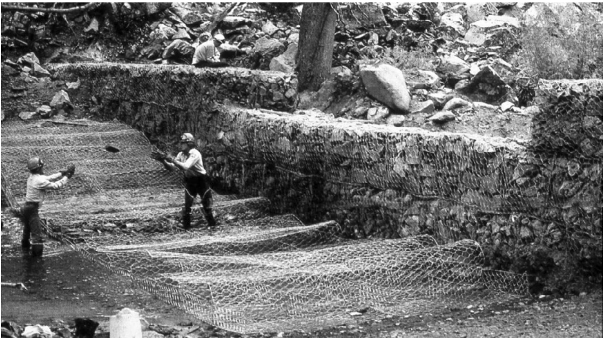
12 - Schaeffer Barrier showing gabion basket construction completed 1983. September 1983. Photo courtesy of INF.
