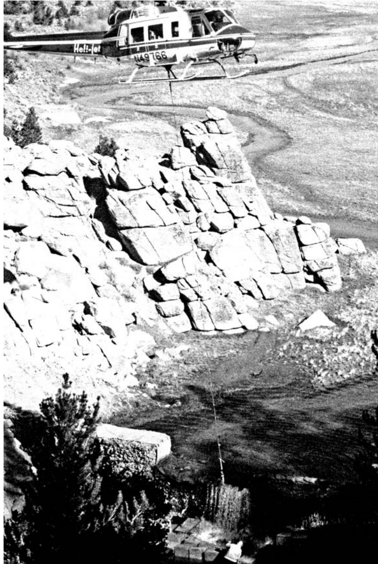
Figure 13 - Helicopter lowering concrete stabilization blocks onto Templeton Barrier apron. October 1988. Photo courtesy of INF.
