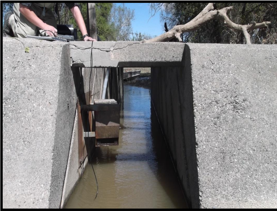
Figure 5. View of Fremont Weir Denil fish ladder after cessation of an overtopping event in March 2016. Note that flash boards have been removed to facilitate fish passage through the weir.
