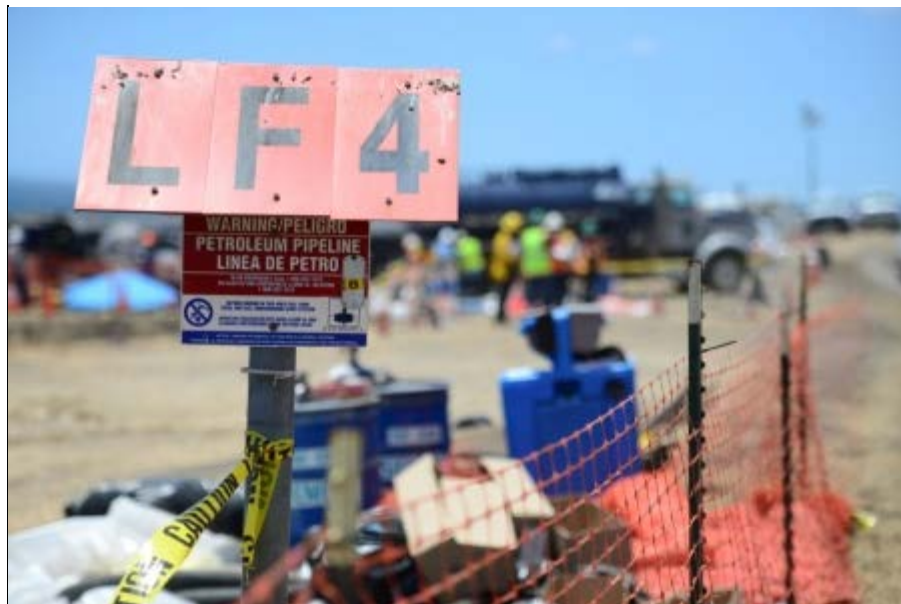
A pipeline marker stands near the point the pipeline released and spilled oil into the environment and eventually into the Pacific Ocean north of Santa Barbara, Calif., May 22, 2015. (U.S. Coast Guard photo by Chief Petty Officer David Mosley.)
