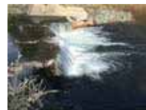
Photo 4-13 Cosumnes River—Blodgett Dam after flood damage /DFG Photo
