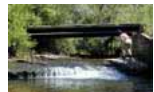
Photo 4-17 Dry Creek— pipeline on Secret Ravine (Sacramento and Placer counties)/DWR photo
