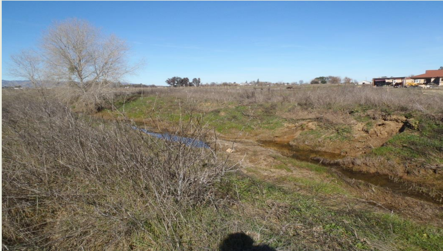
Bank sloughing and lack of riparian vegetation on Dry Arroyo (Facing north)
