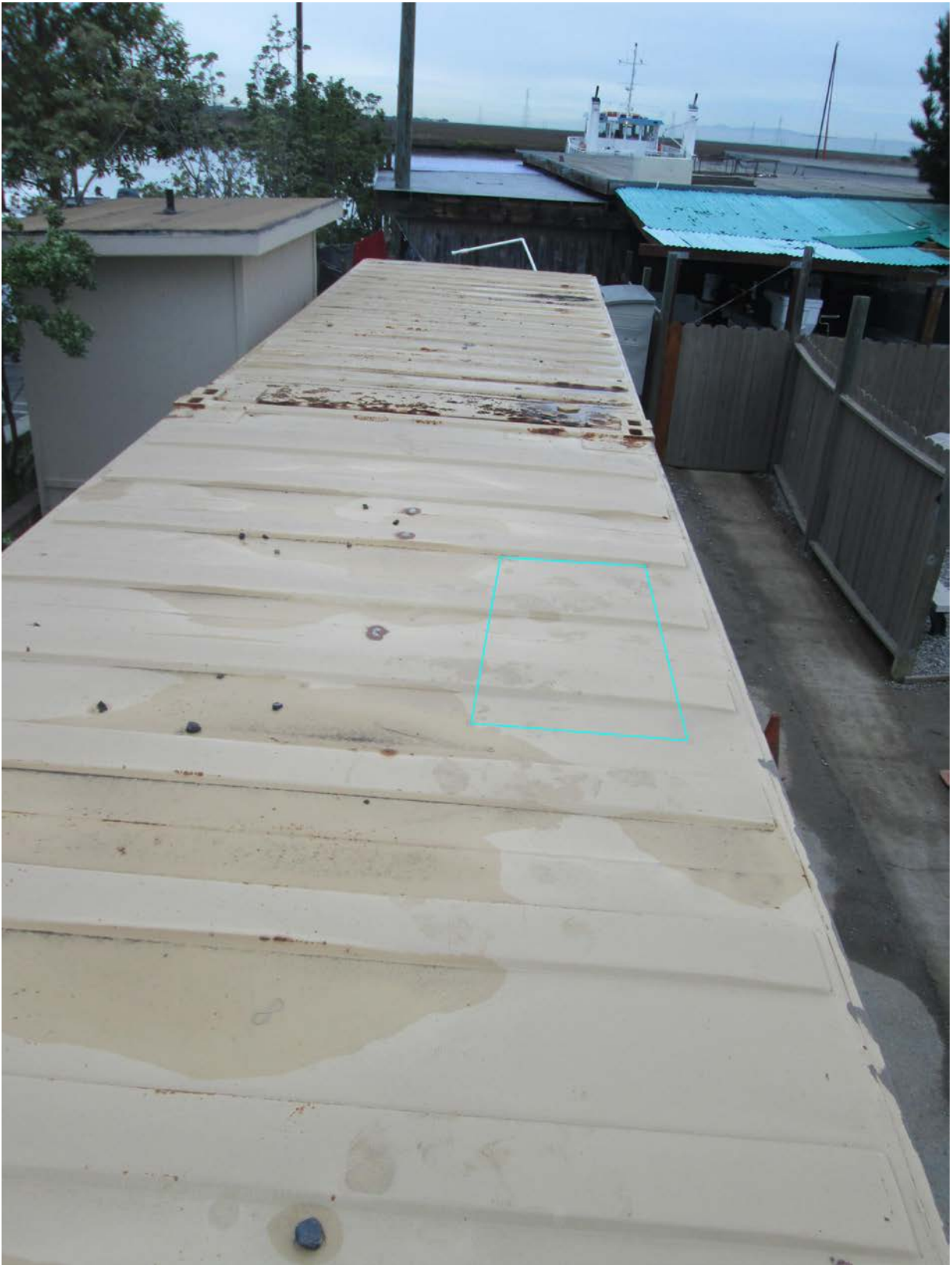
Photograph 7: Photo of the roof of the restrooms and where the skylight will be placed (BEFORE PROJECT). (Photo by Jesus Jimenez)
