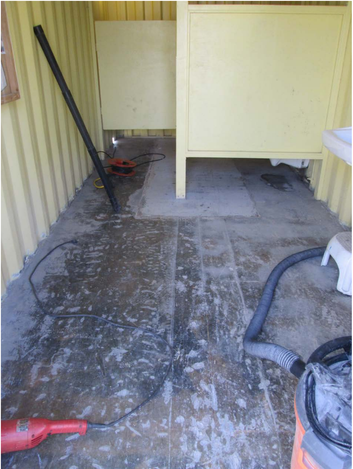
Photograph 4: Photo of flooring in women's room, before new durable Epoxy flooring was installed. Also shows old wooden partitions and old paintwork (BEFORE PROJECT). (Photo by Jesus Jimenez)
