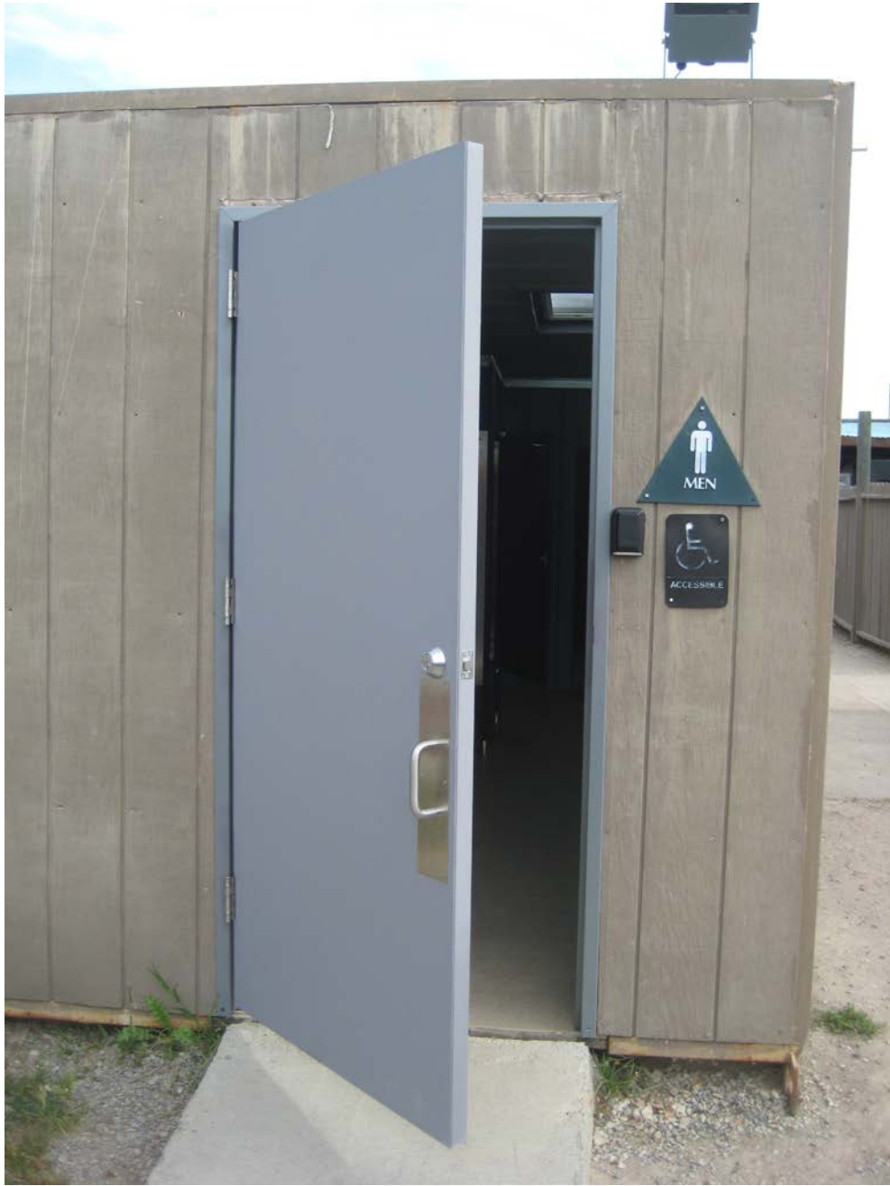
Photograph 3: Outside view of men's room showing new industrial locking door (AFTER PROJECT). Not shown: same style door at entrance to women's room. (Photo by K.C. O'Shea)
