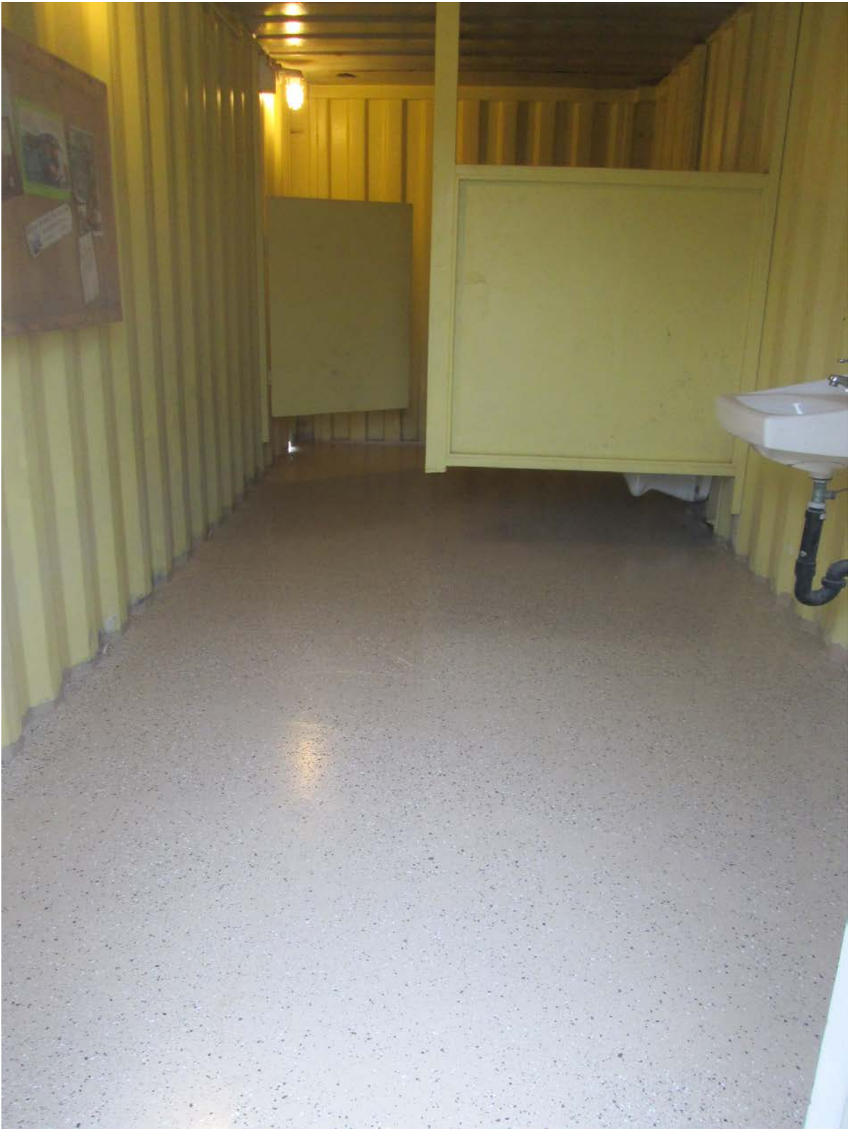
Photograph 5: Photo of newly installed Epoxy flooring (AFTER PROJECT). (Photo by Jesus Jimenez)
