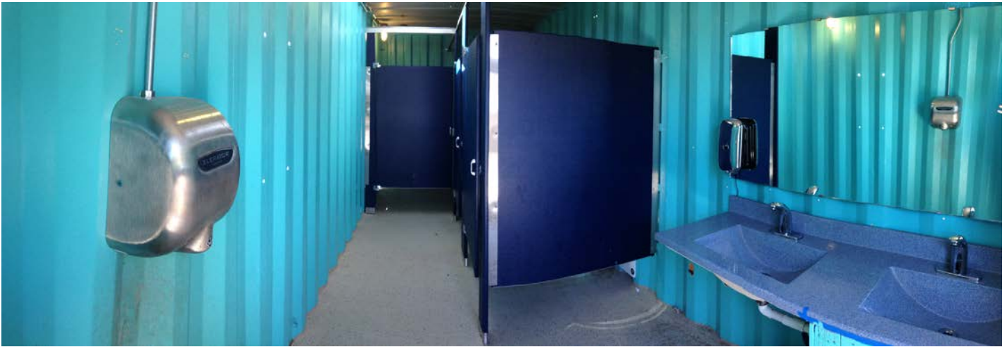
Photograph 1: Panoramic view of the women's restroom showing the paintwork, new partitions, new hand dryer, new third stall, double basin sink, automatic soap dispenser, and epoxy flooring (AFTER PROJECT). (Photo by K.C. O'Shea)
