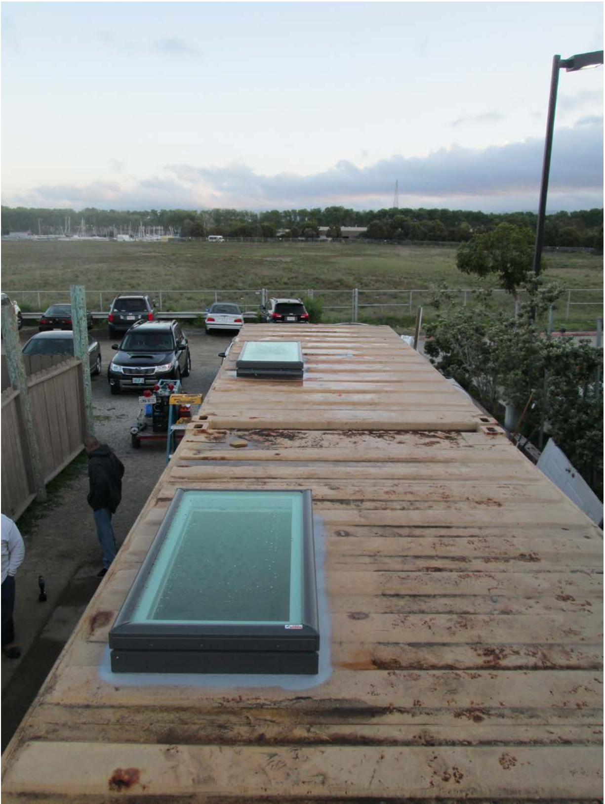
Photograph 8: Photo of the newly installed, solar-powered skylights (AFTER PROJECT). (Photo by Jesus Jimenez)
