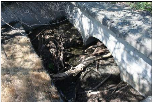
Figure 19: Hwy 101 Culvert 21 full of debris.
