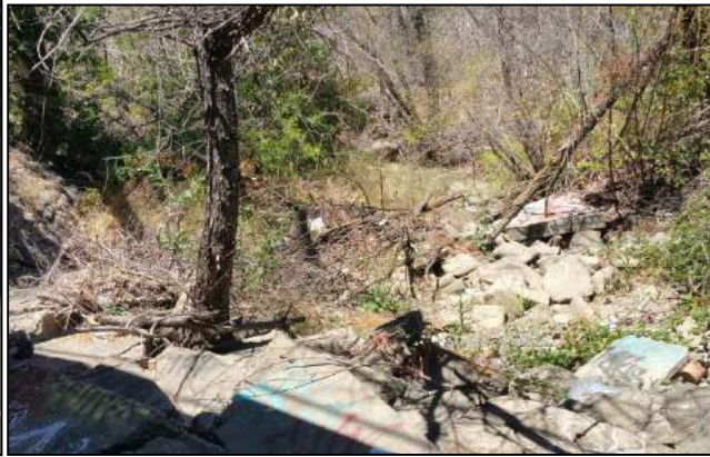
Figure 21: Debris at Monterey Road Culvert.
