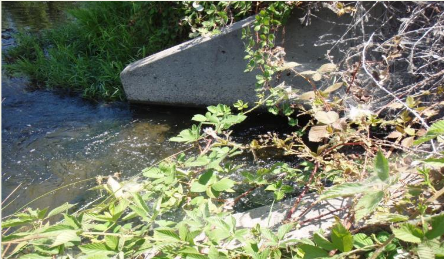
Existing storm drain outfall in secondary channel of the San Joaquin River
