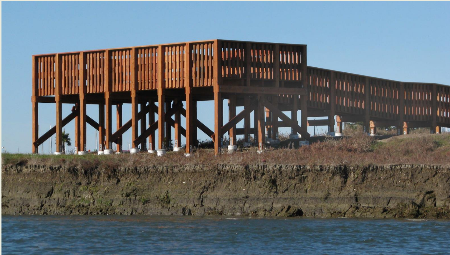
Western Observation Platform close up showing bank erosion
