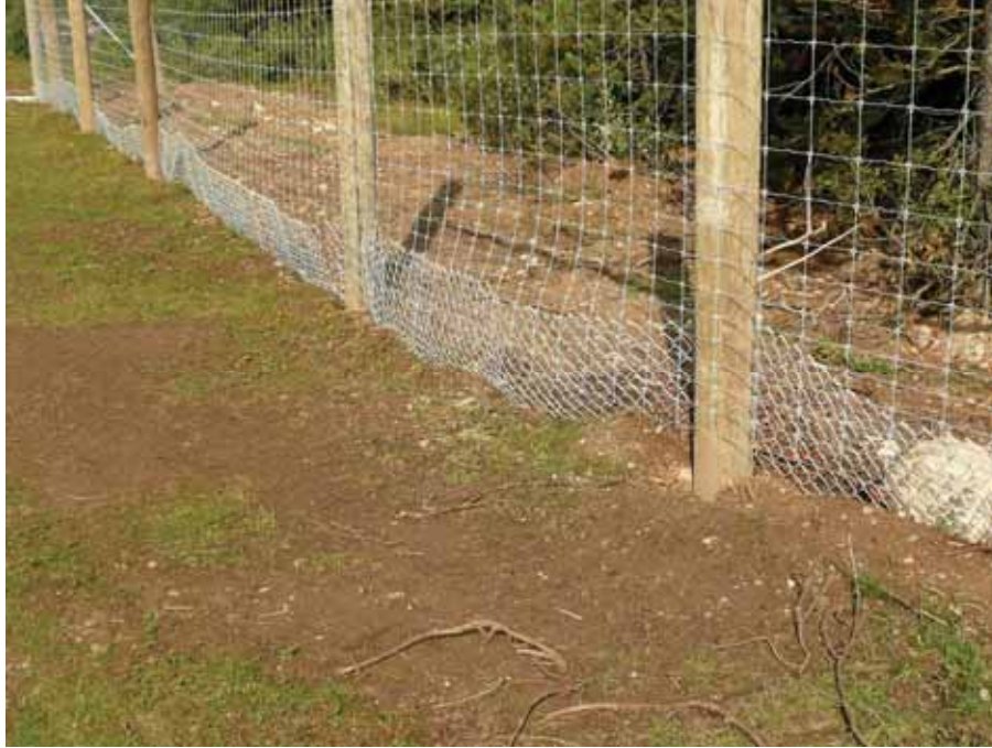
Figure 65. Photo. Wildlife exclusion fence with buried apron (Credit: Tony Clevenger).
