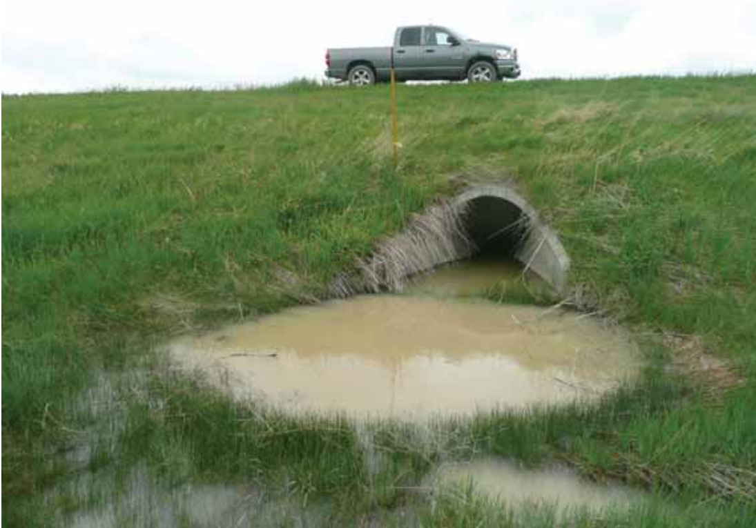
Figure 58. Photo. Flooding in front of tunnel due to improper drainage design (Credit: Tony Clevenger).
