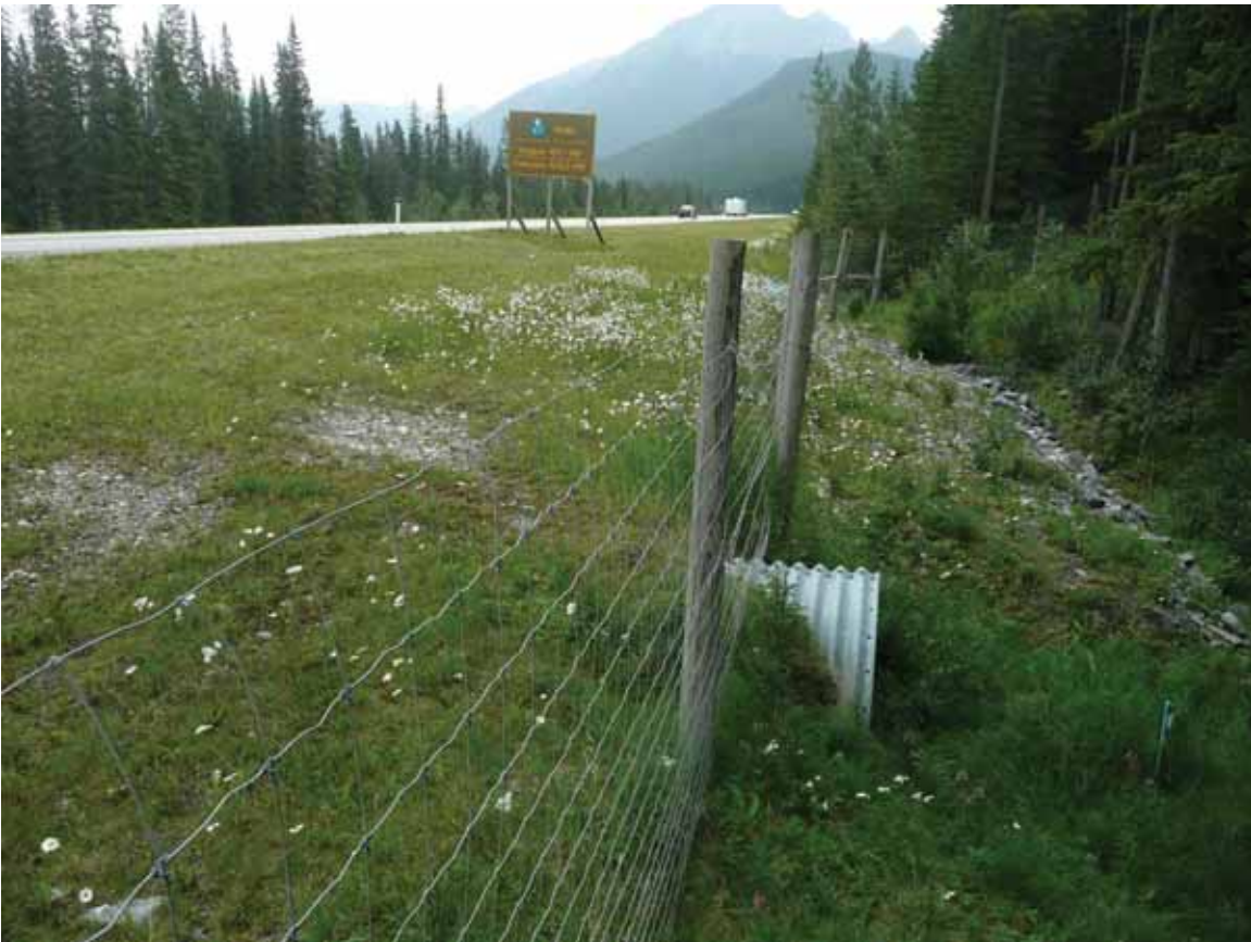
Figure 62. Photo. Wildlife exclusion fencing and culvert design wildlife underpass (Credit: Tony Clevenger).
