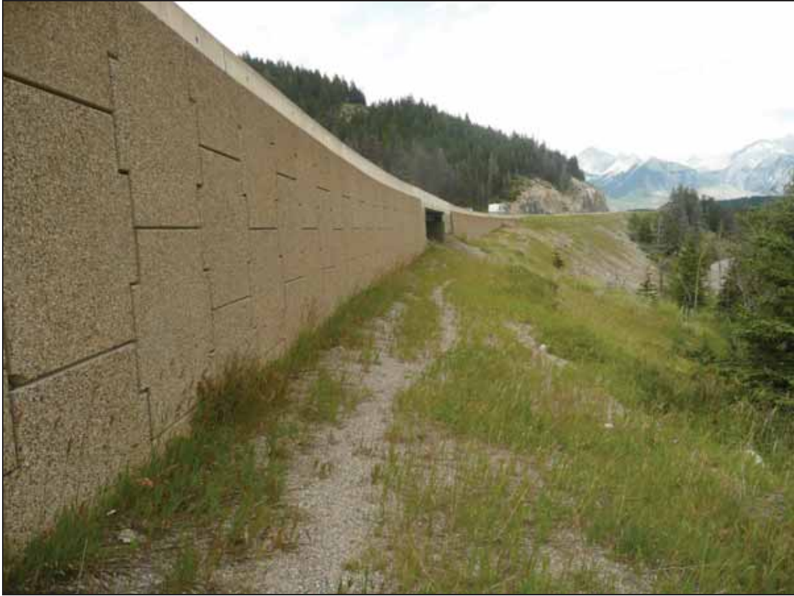
Figure 47. Photo. Mechanically stabilized earth (MSE) wall serving as wildlife exclusion “fence” (Credit: Tony Clevenger).
