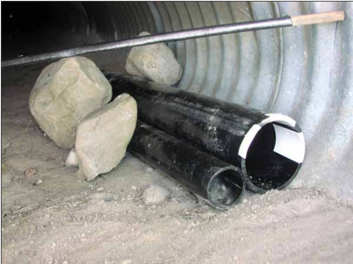
Figure 48. Photo. Pipes placed in culverts to provide cover for small mammal movement (Credit: Tony Clevenger).
