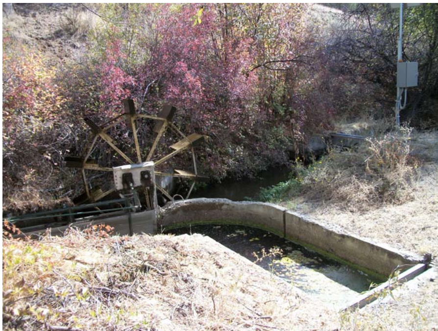
Site HR02. Roll Hart-01, Frame 07. Overview of south end of diversion structure. Diversion ditch is to right of water wheel. Flow meter and solar panel is at far right. View 160 degrees.
