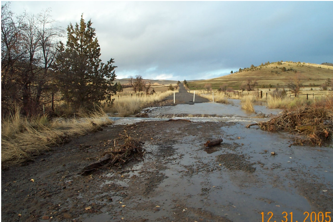
Photograph 1. 2005 Post Flood Photograph Harry Cash Road (700 ft North of Bridge)
