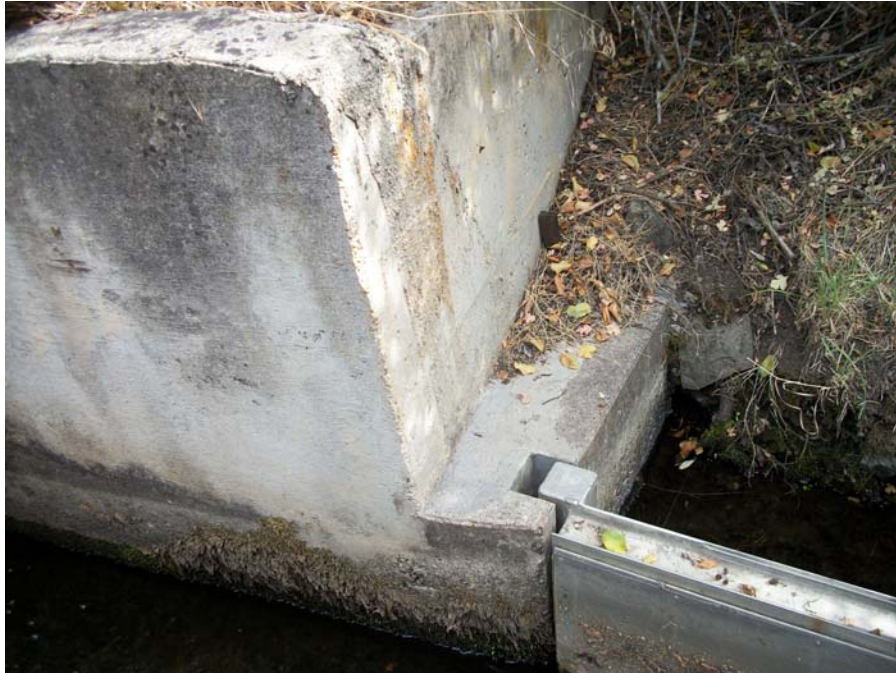
Site HR02. Roll Hart-01, Frame 13. Closeup showing concrete work and where the fish screen is anchored to it. View 104 degrees. 9/30/2016.
