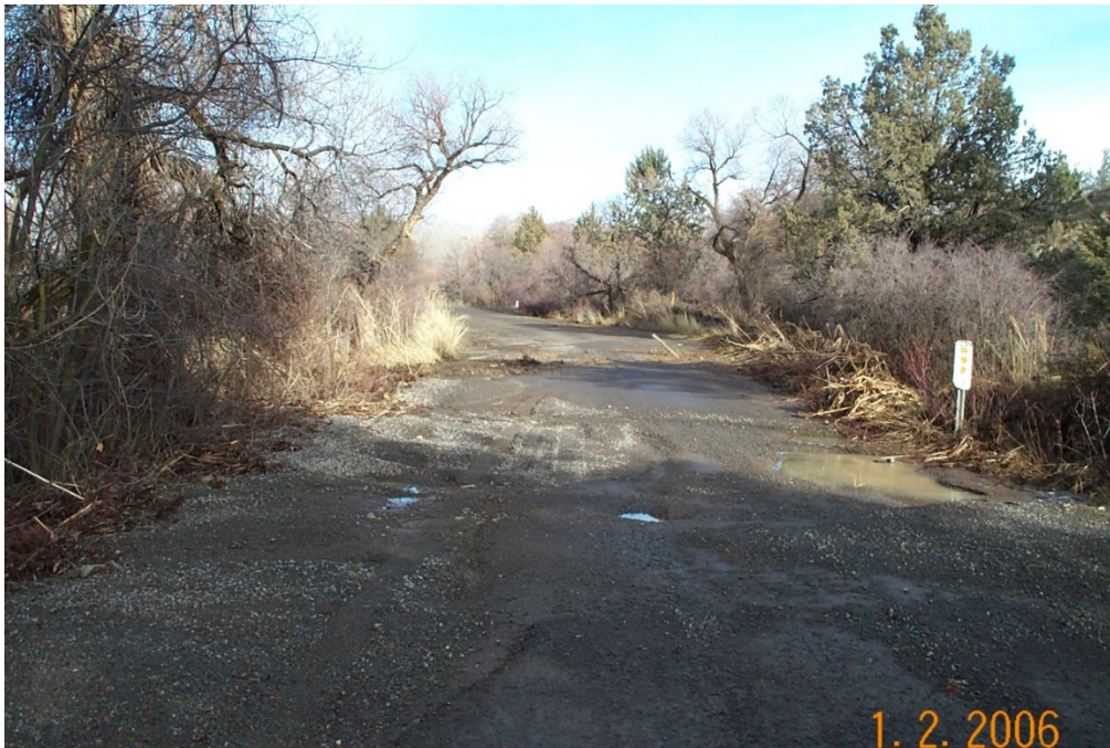
Photograph 3. Post Flood 2005 Flood Harry Cash Road (200 feet south of the Bridge)
