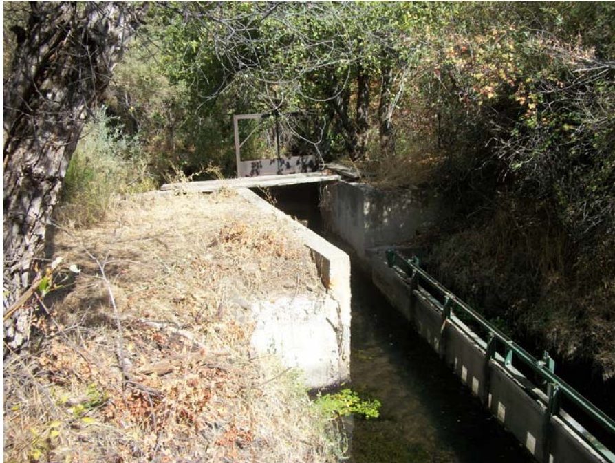
Site HR02. Roll Hart-01, Frame 08. View of diversion structure with fish screen on right and headgate in background, middle. View 170 degrees. 9/30/2016.
