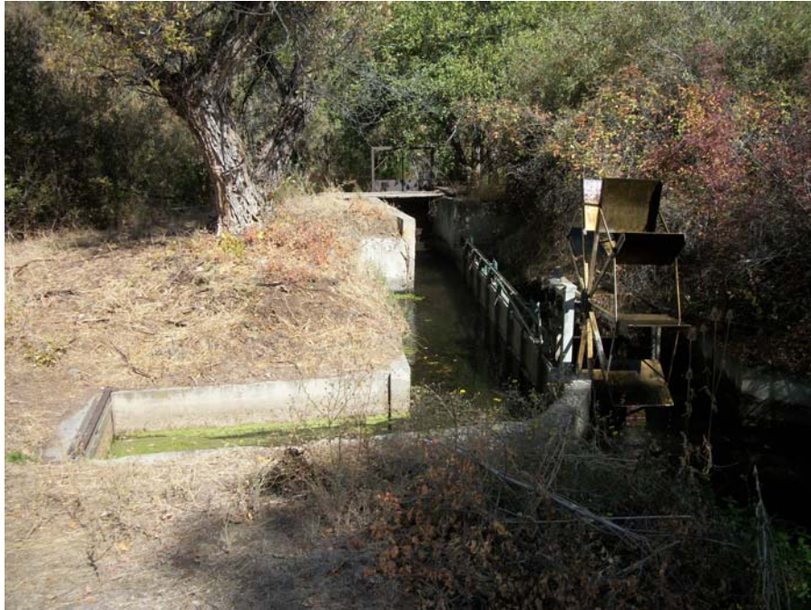
Site HR02. Roll Hart-01, Frame 06. Overview. Shows diversion structure with concrete retaining walls, undershot water wheel (allows for mechanical cleaning of fish screen), fish screen, and headgate. View 64 degrees.
