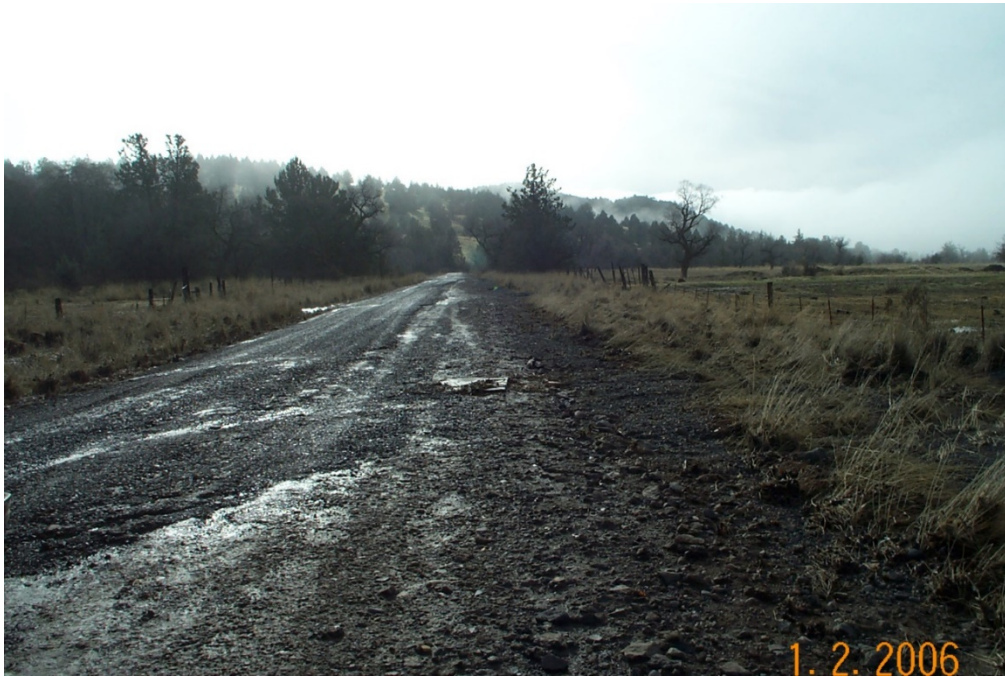
Photograph 2. 2005 Post Flood Harry Cash Road (700 ft North of Bridge)
