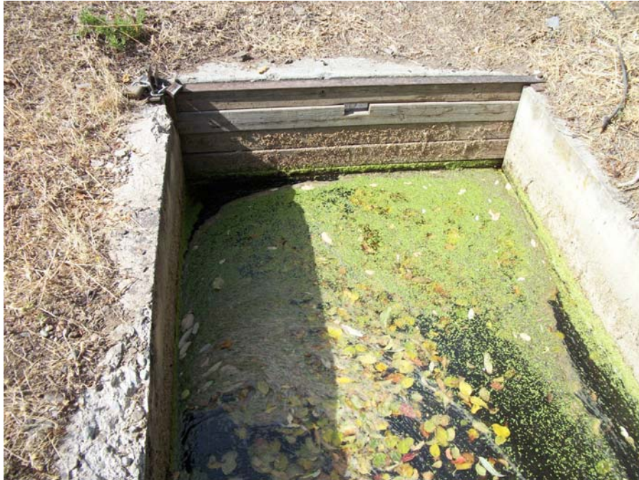
Site HR02. Roll Hart-01, Frame 15. View of overflow channel. Flows into a pipe just below the water surface. This pipe was likely the fish return pipe. View 318 degrees. 9/30/2016.
