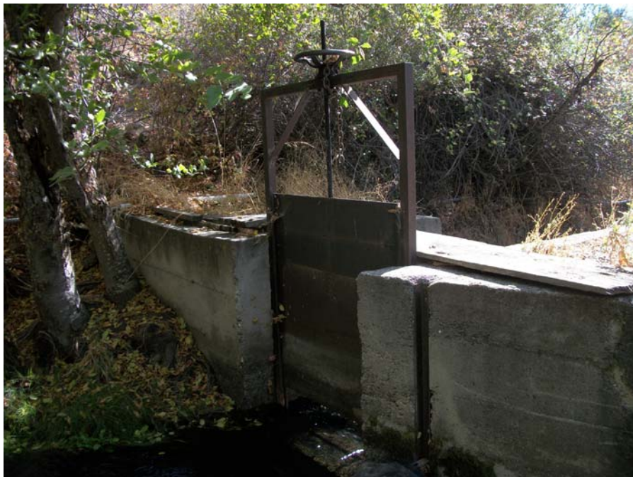
Site HR02. Roll Hart-01, Frame 09. North end of diversion structure showing concrete work, headgate, and wheel. Milled lumber forms were used when this part of the structure was built. View 164 degrees. 9/30/2016.
