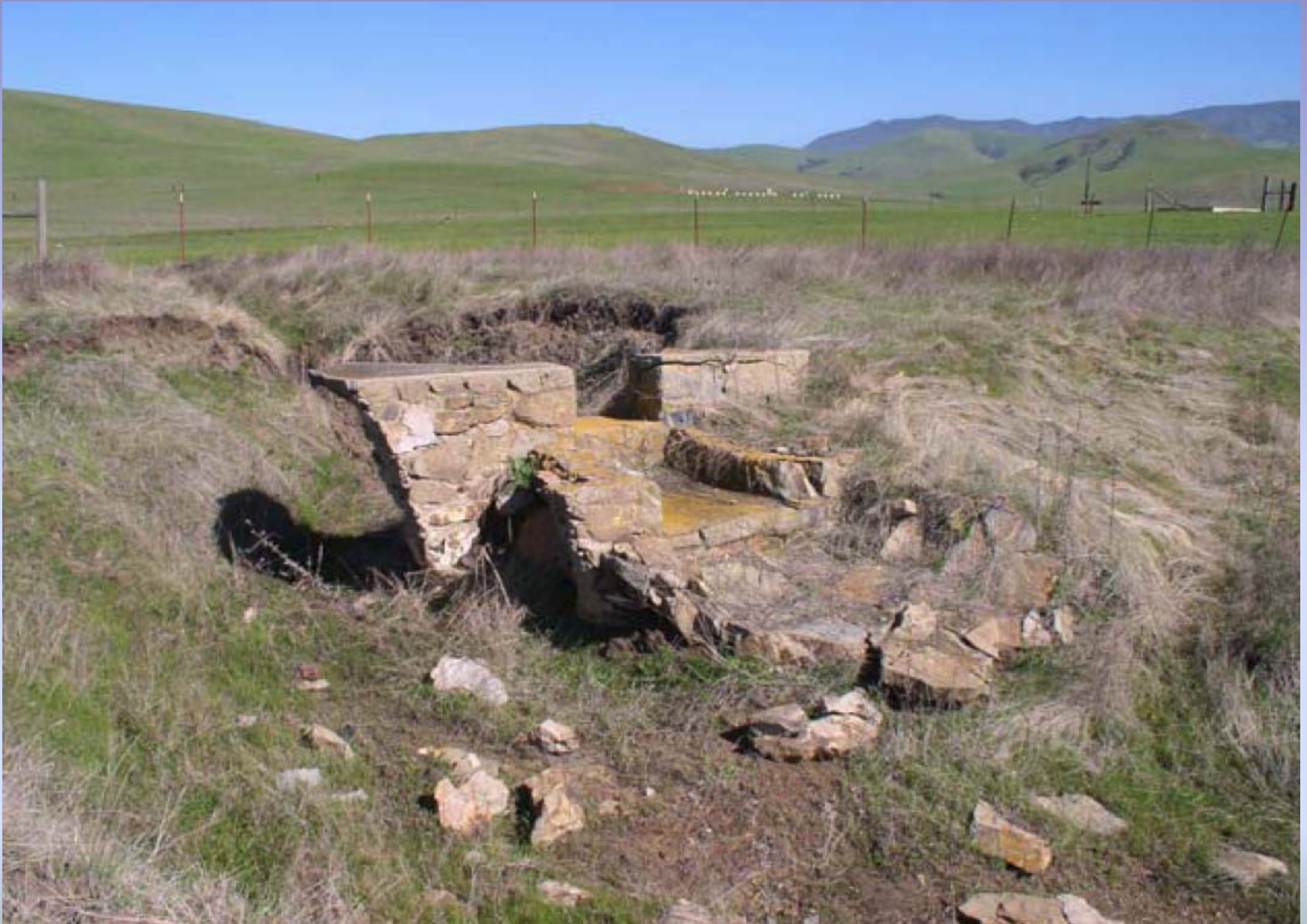
Failed Grade Control Structure on Tributary – Site 2
