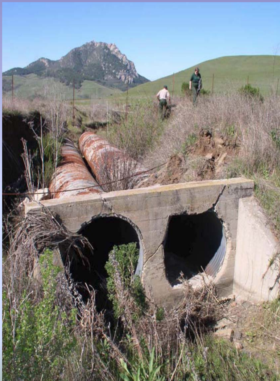
Failed Road Crossing – Site 2
