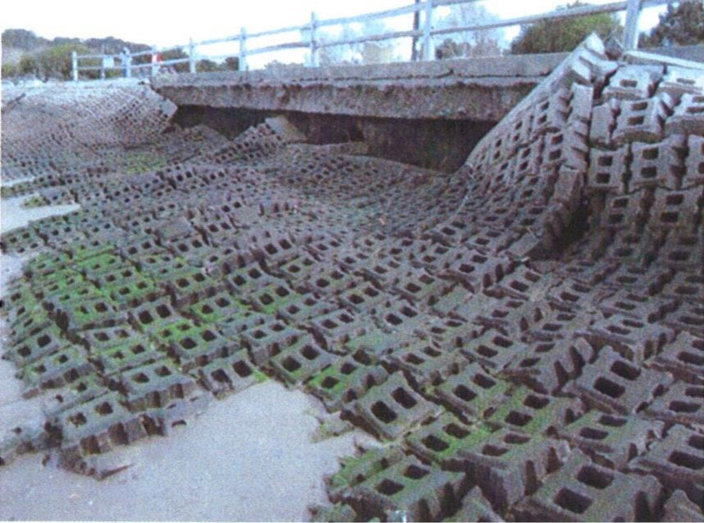
Image 1: Photo shows failed shoreline armoring prior to the project. Concrete blocks have separated from the Promenade pathway. Public access ramps for watersports are neither safe nor easy to use.
