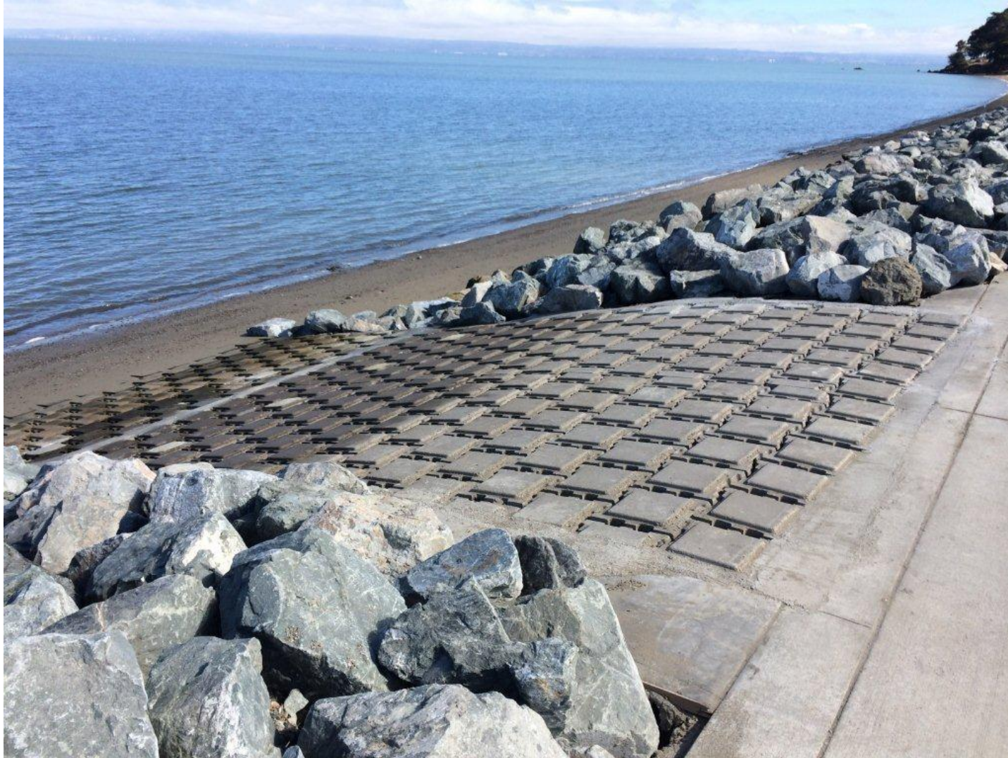
Image 4: Well-engineered access ramp is shown (post-project). The ramp has interlocking blocks, is flush with Promenade trail, is built down to the bay mud, and is well defined amidst the revetment.
