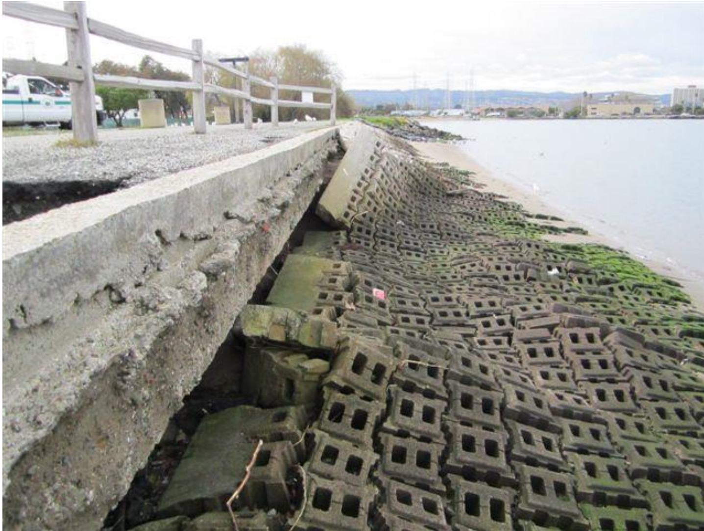
Image 2: Photo shows buckling of public access ramps and lack of revetment prior to the project.
