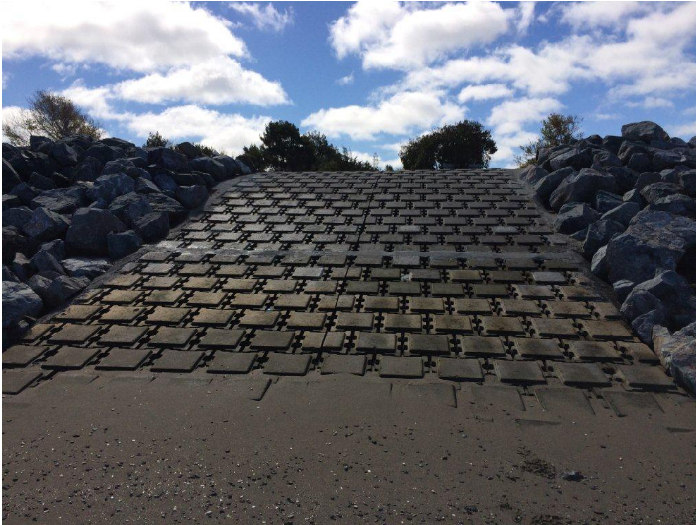
Image 6: View of new access ramp from Bay at low tide (post-project). Shows easy access from the Bay to the Promenade for recreational users who carry boats, boards and sails.
