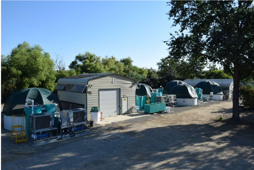
Figure 23: Interim Facility with water recirculating and water chilling enhancements.
