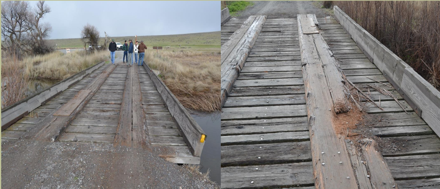
Damage and old repairs to the entrance bridge
