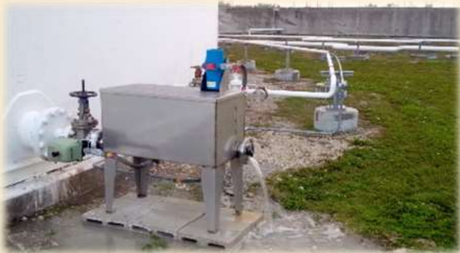
EnviroEye System in Operation at Naval Air Station (photos courtesy Pipeline & Terminals Management Corp - PTMC)
