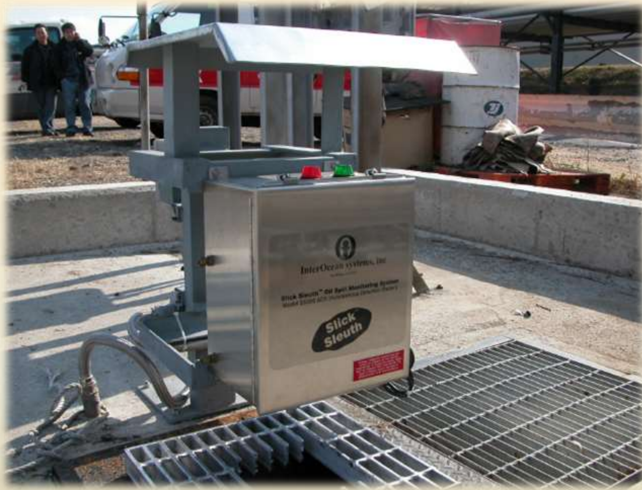
Autonomous Spill & Leak Detection Monitoring for Oily Discharge in Industrial Storm Water Sewer (photo courtesy SK Energy)
