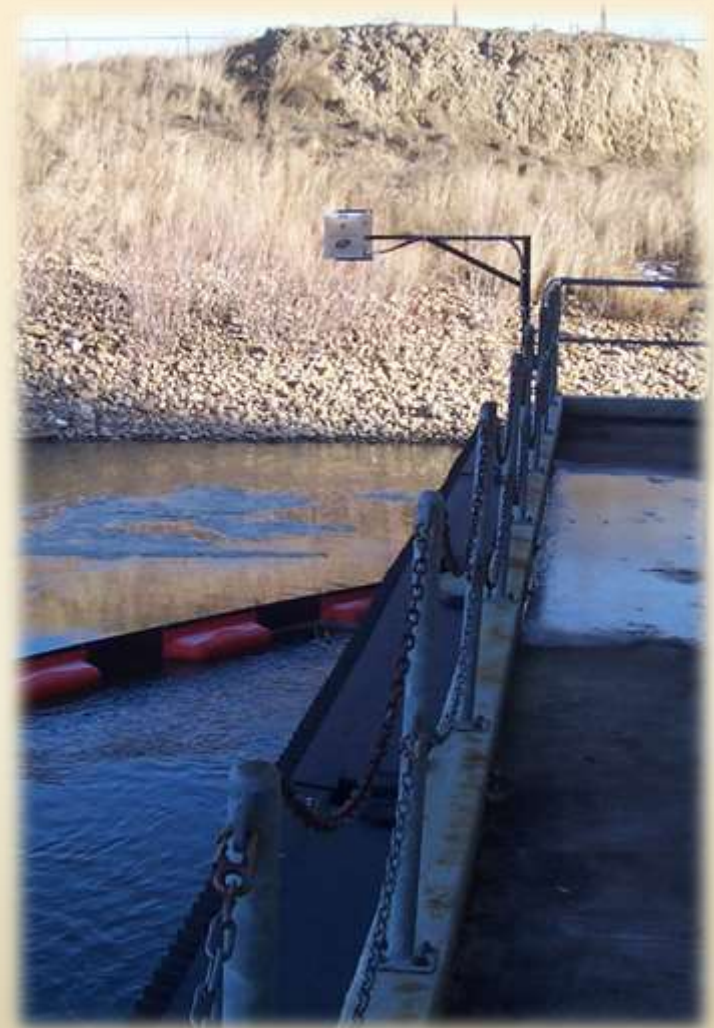
Power Plant – Cooling Water Discharge / Outfall (note positioning of fixed-containment boom below sensor)
