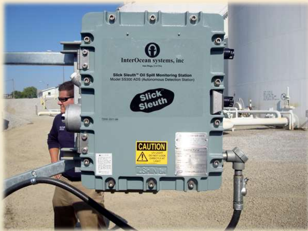
Monitoring for Leaks/Spill within Secondary Containment Above Ground Storage Tank (AST) Facility
