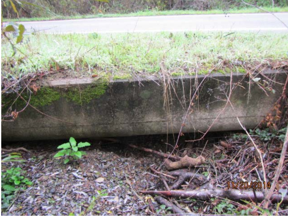
Figure 10. Sediment accumulation in culvert at MRN 1 14.86. Upstream looking downstream. November 2014.
