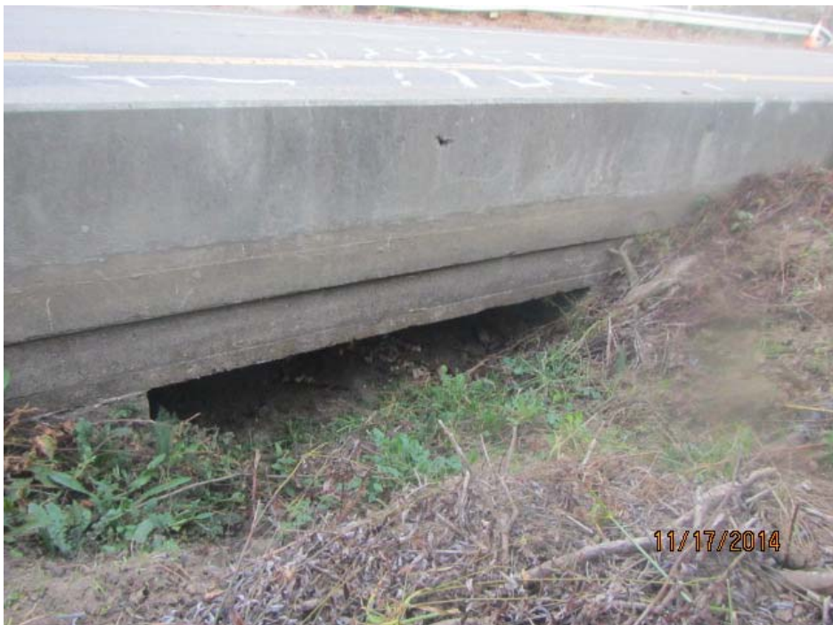
Figure 11. Sediment accumulation in culvert at MRN 1 27.92. Downstream looking upstream. November 2014.
