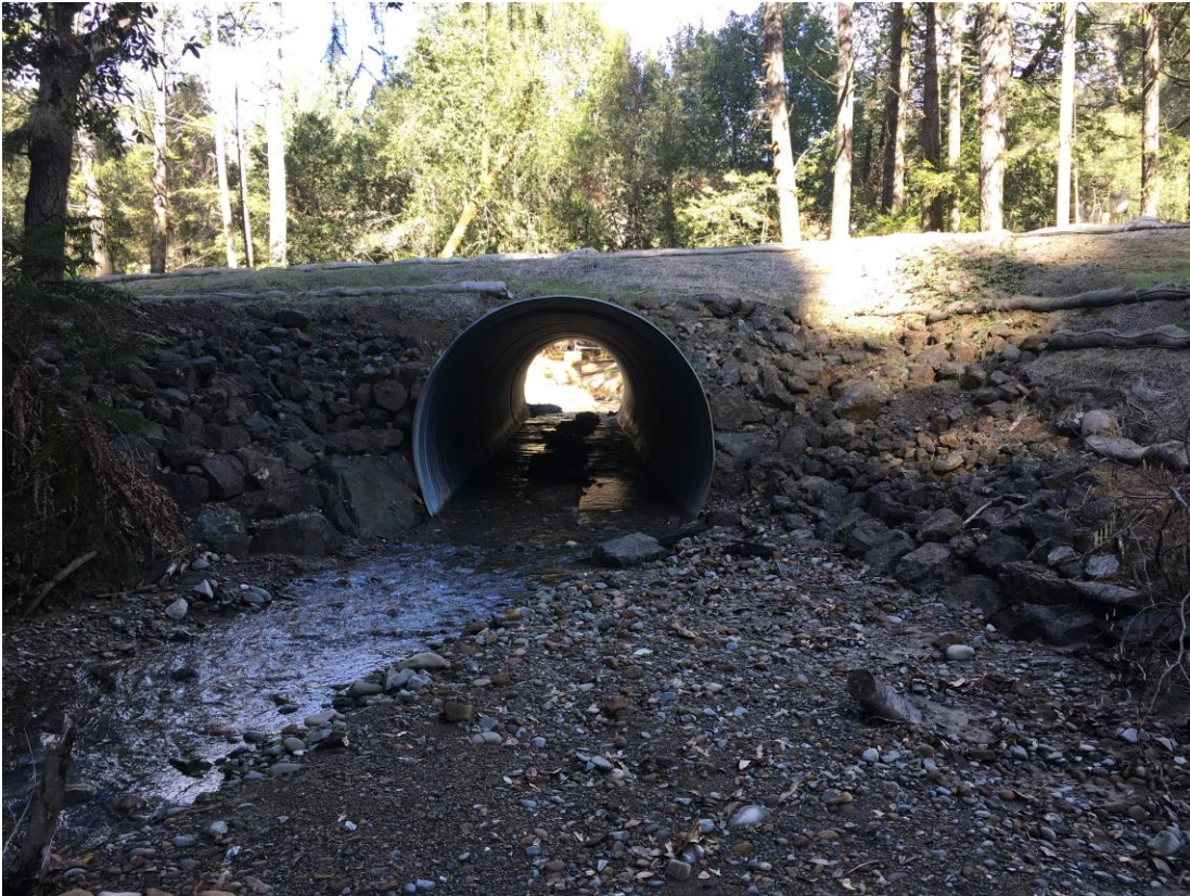
Picture 1. Looking upstream at Briceland Thorn Road crossing replaced during winter 2016/2017. PAD ID 713215.
