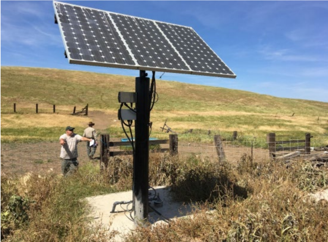
Image 5: After – solar panel installation at the project site located at the base of an old windmill pump that was cleaned up. The restored cattle well is located behind the black pole mounting the solar panel.
