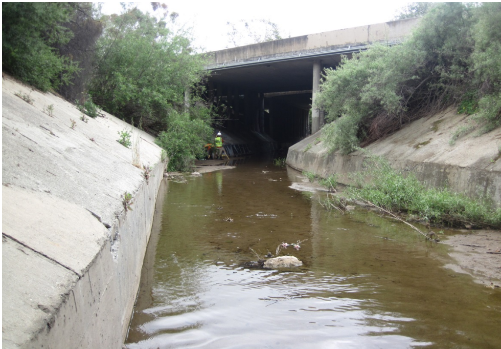
Photo 5. Route 101 (PM 21.63), San Jose Creek, looking upstream at concrete walls throughout survey site.
