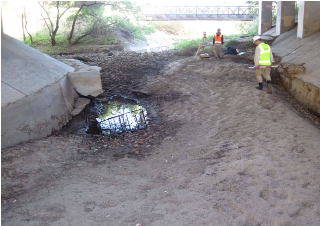
Photo 3. Route 101 (PM 20.95), looking upstream at the confluence of Maria Ygnacio Creek and San Antonio Creek.
