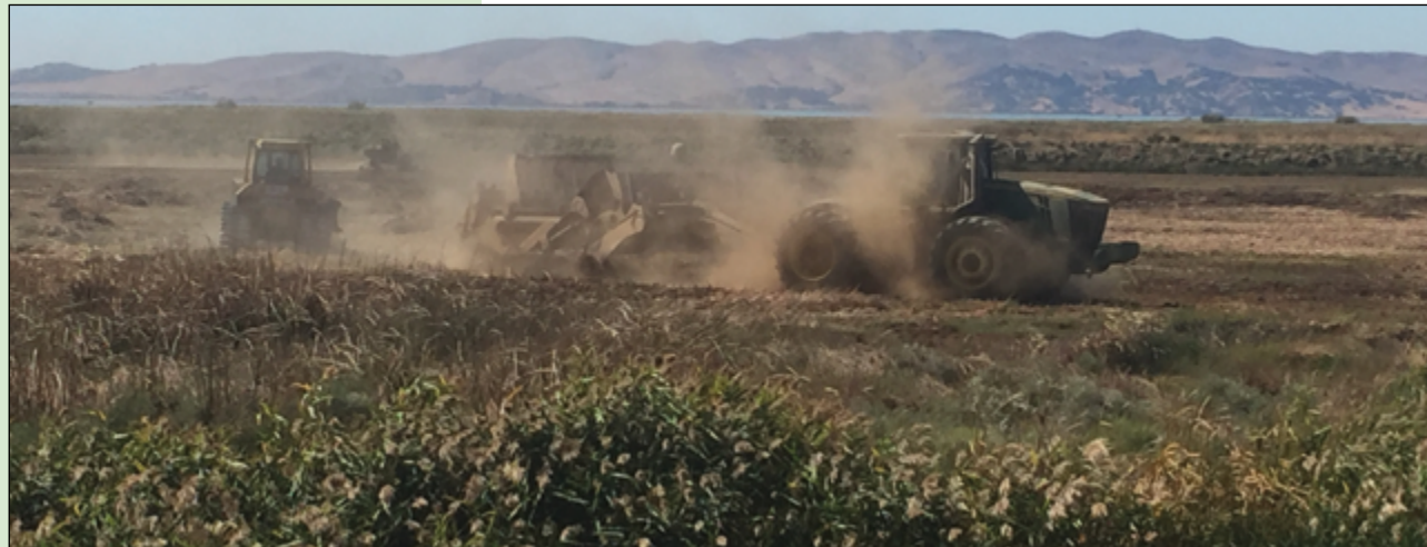
Low pressure grade tractors, cats, dozers, and scrapers laying the groundwork for restoring tidal action to the Tule Red property in Suisun Marsh. Photo: Westervelt Ecological Service
