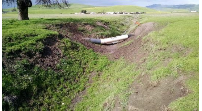
Photo 24. Pipeline span across the channelized portion of Cayetano Creek within the action area. Taken facing N. (2/19/16)
