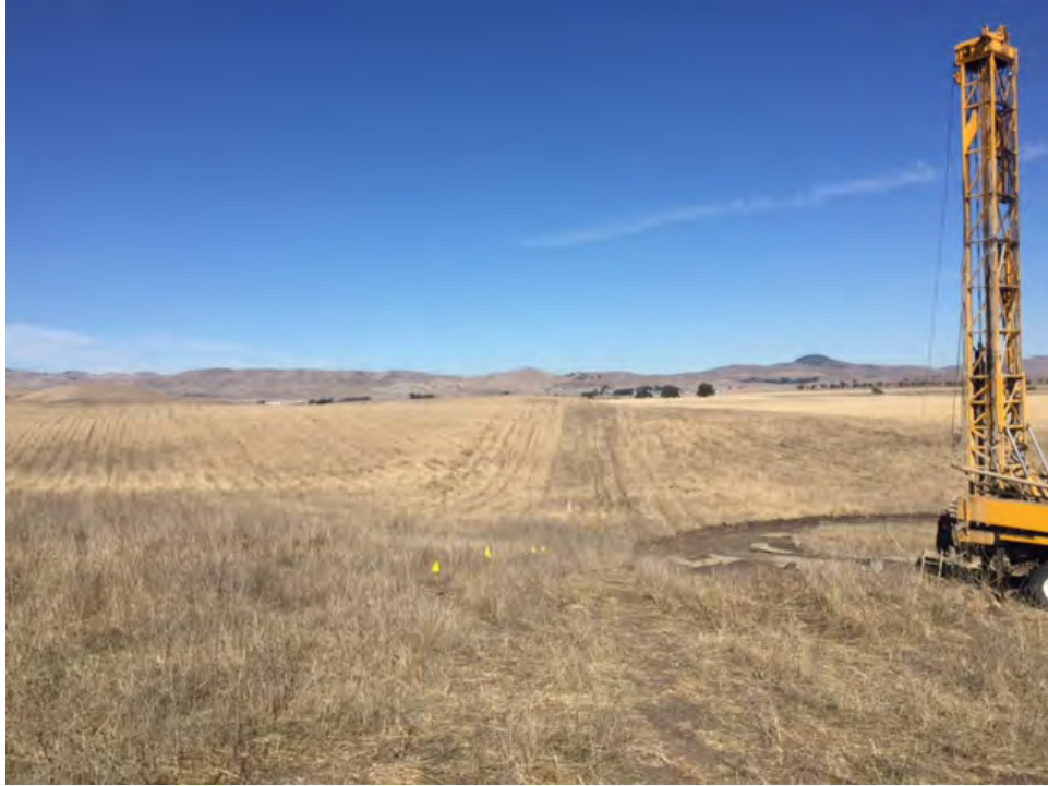
Photo 0988: View to well-drilling equipment just east of the pipeline alignment, just east of the small, square staging area where the access road and the alignment intersect. View Towards the North. Photographed by Joanne Grant on 10/20/2016.
