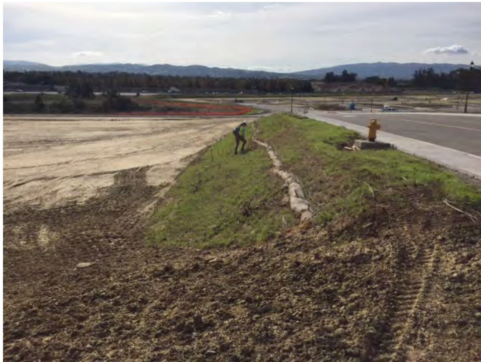
Photo 1022: View from the northeastern portion of the project area, just south of Portola Ave, from top of berm. View is toward the South. Photographed by Joanne Grant on 11/7/2016.
