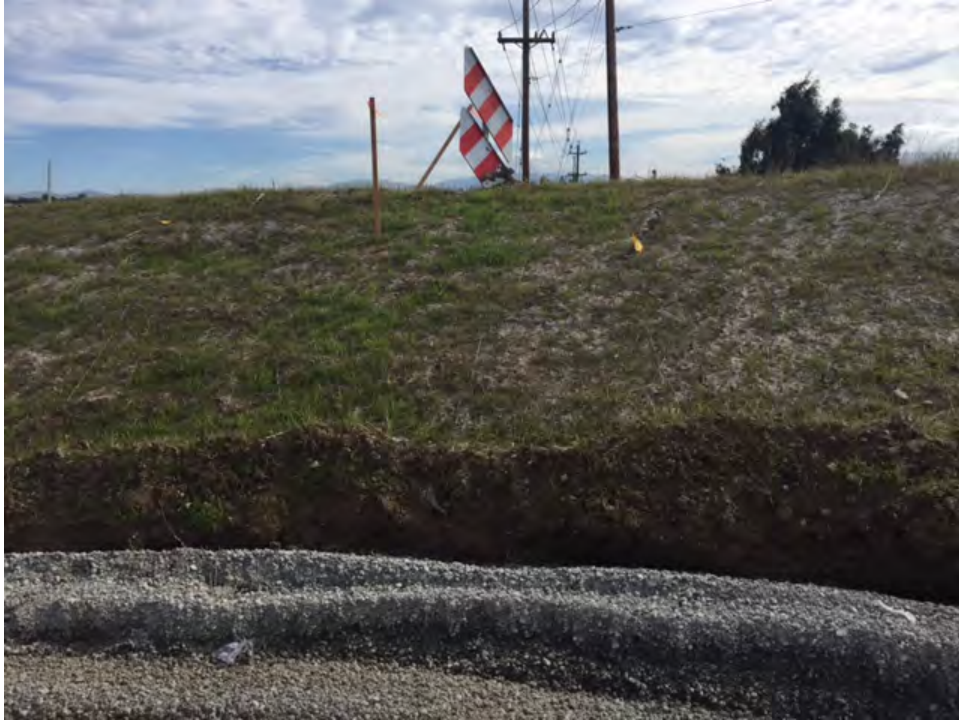
Photo 1019: View to the berm, showing the flags indicating the buried pipeline, and imported fill. View Towards the Southeast. Photographed by Joanne Grant on 11/7/2016.
