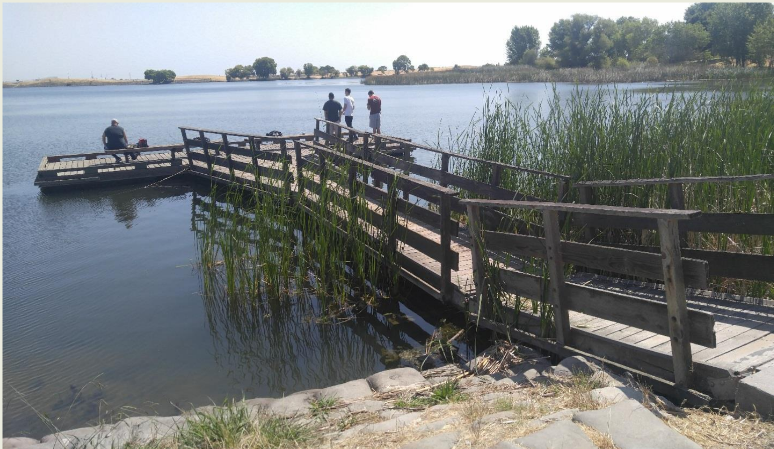
The Deteriorated Channel Point Fishing Dock before closure.
