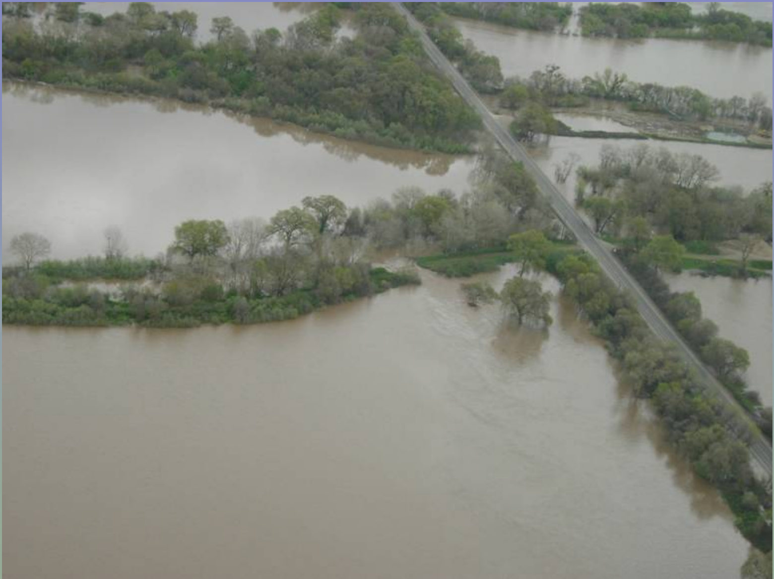
Close up of Denier and Oneto II properties in April of 2006 showing levee breach
