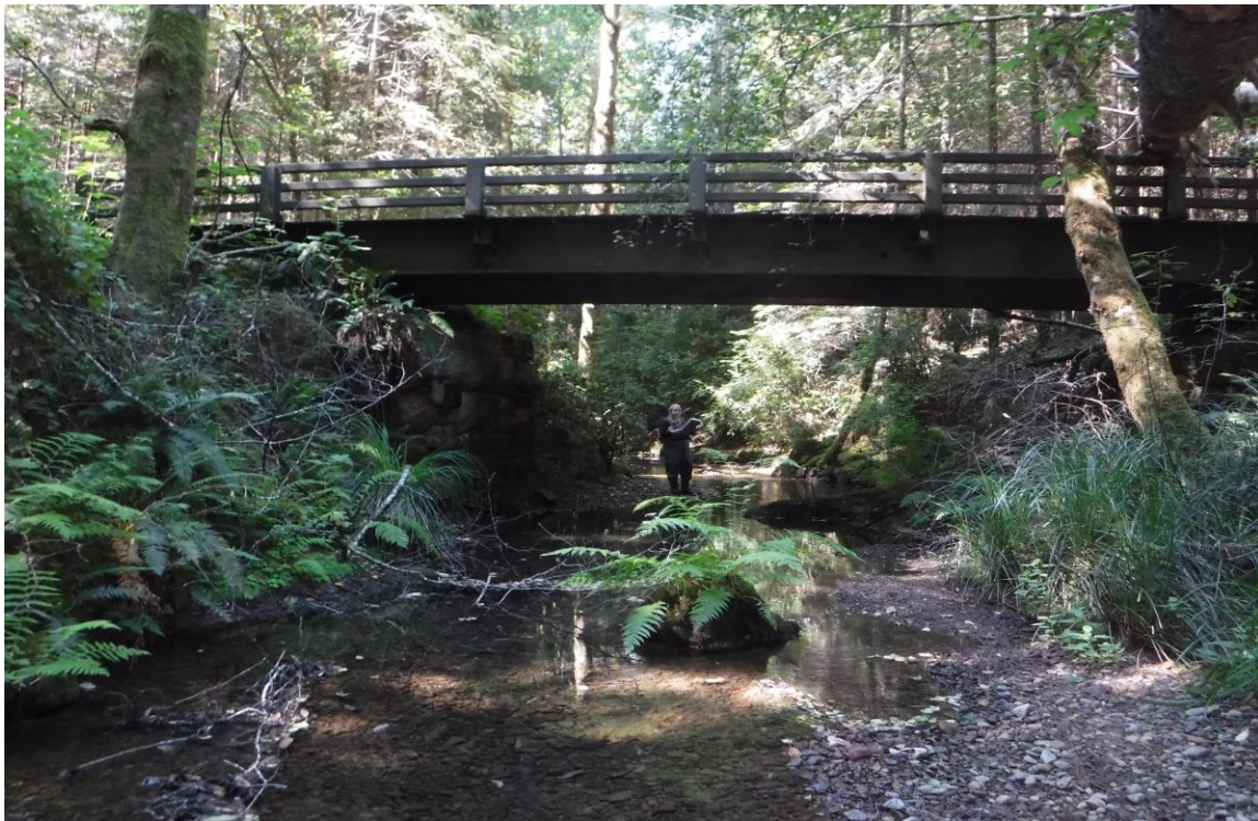
Photo 3: Bridge #1 at habitat unit #340; 22,683' upstream of start of survey. Looking downstream Pictured: Kori Roberts. (Photo taken 8/2/17)
