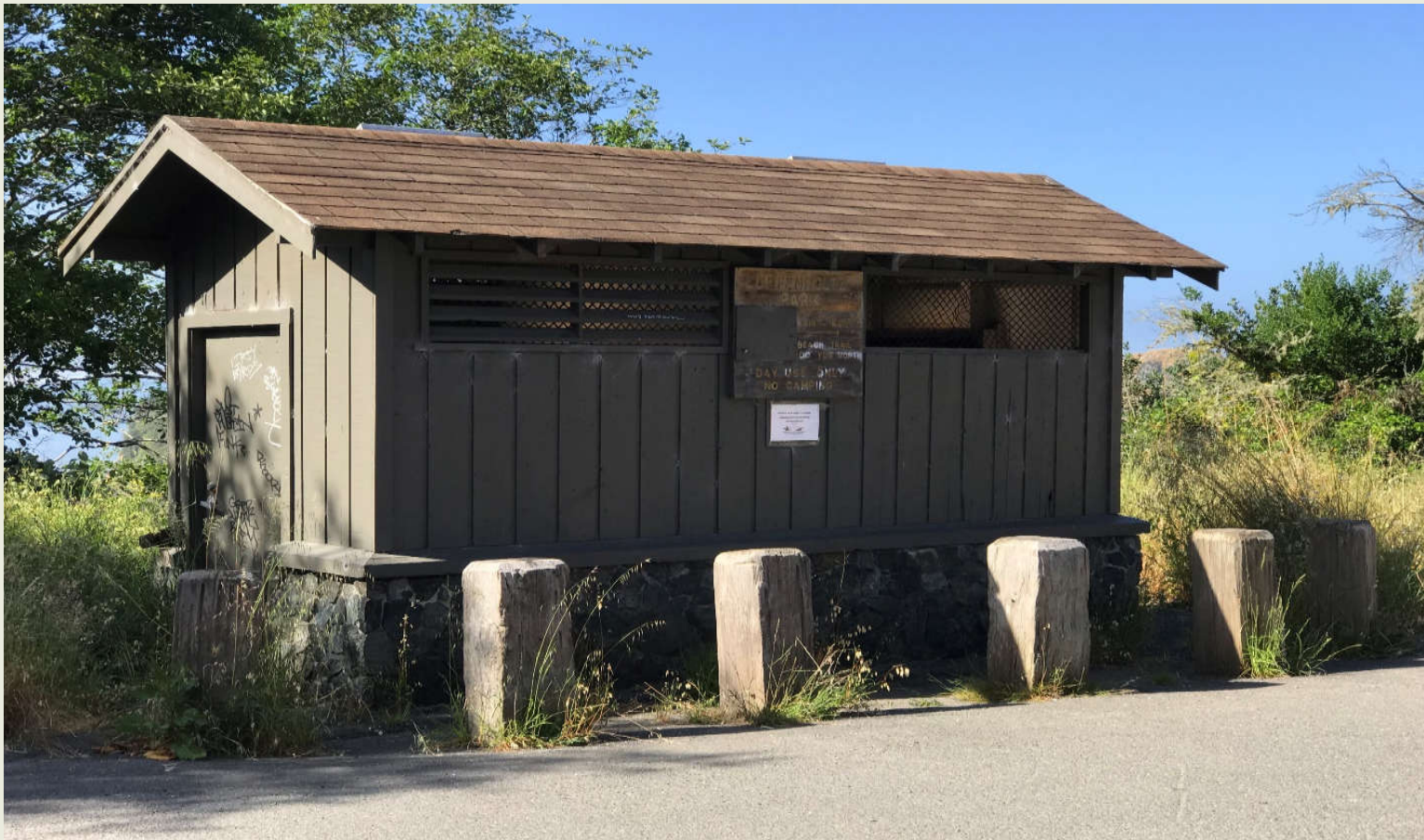
Closed dilapidated restrooms
