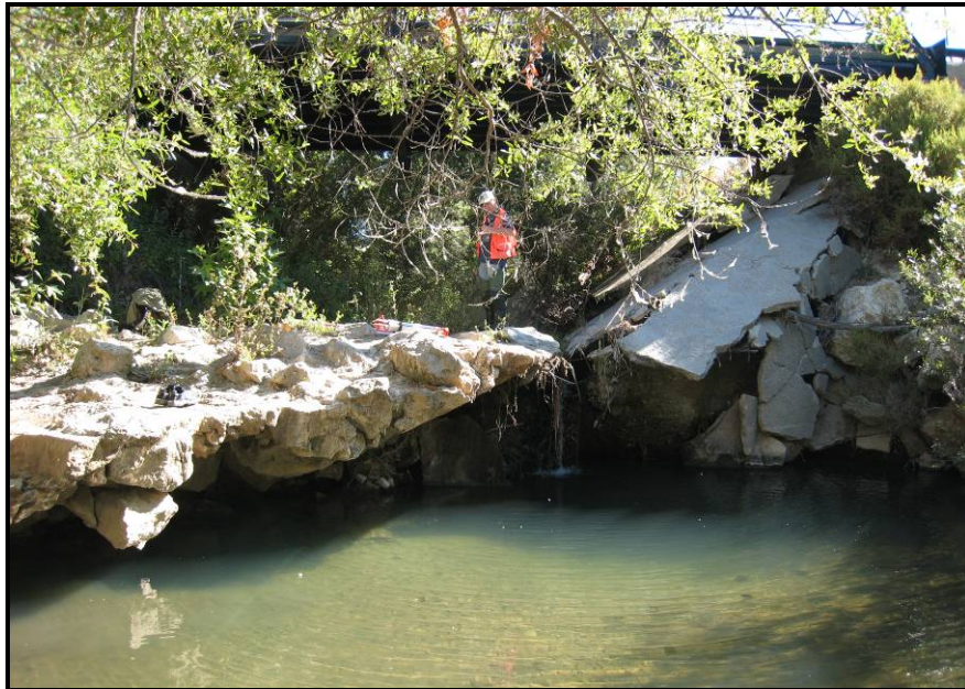
Figure 2 – Looking upstream at the State Park Bridge at San Julian Road. Note undercut broken concrete and grouted riprap within the active channel. The concrete spans the channel and ponds water upstream of the crossing.
