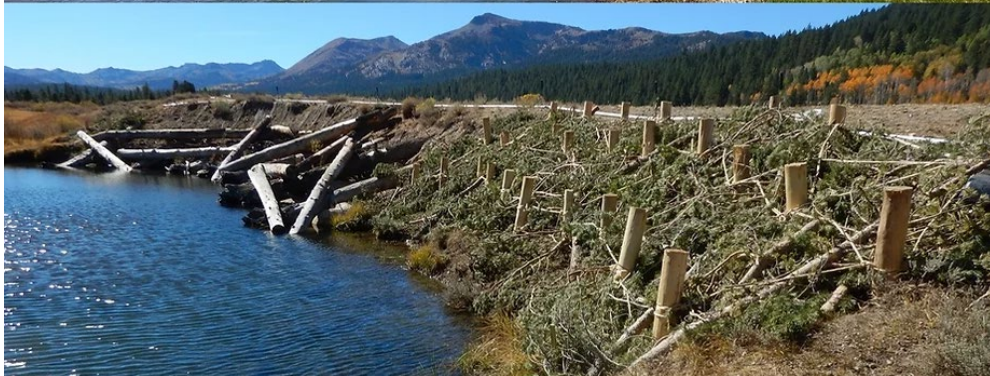
Project Site 2 before (above) and after construction (below) - updates were needed to divert stream energy from scouring behind the 2015 log crib structure so slash was installed at the ends of reach to add stability.
