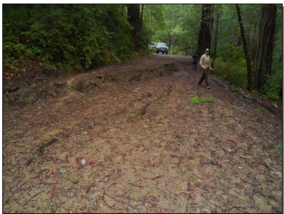
Figure 35. Example of legacy road failure in SF Eel River Basin.
