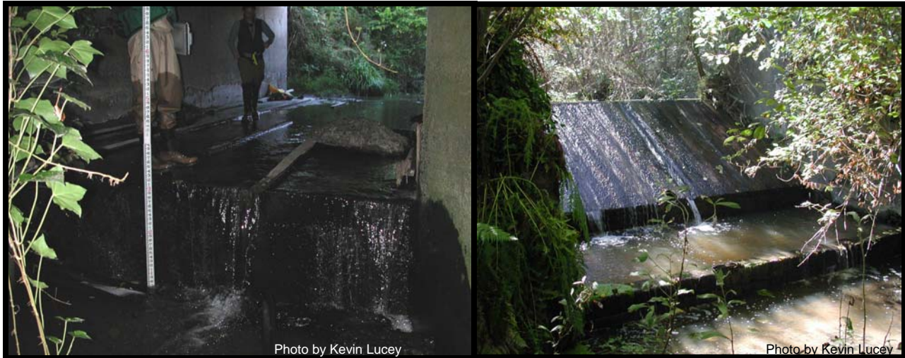
Figure 31. Centerville Road culvert on Russ Creek (left) and fish barrier on Russ Creek 500 ft. above Centerville Road (right).
