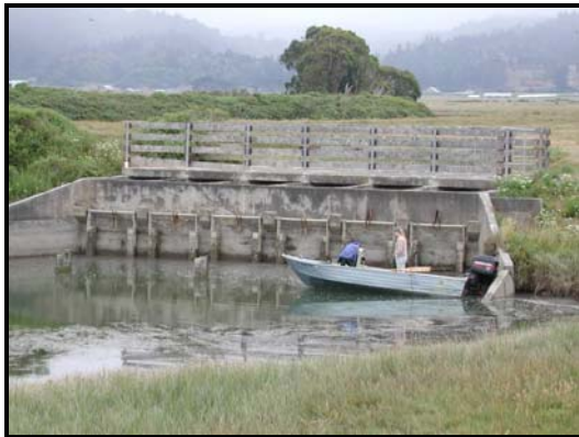
Figure 40. Tide gate on Cutoff Slough.
