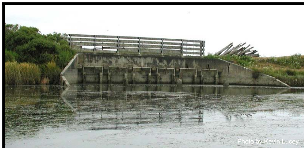
Figure 8. Cutoff Slough tide gate
