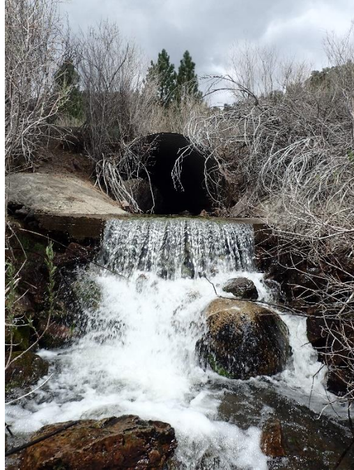
Culvert and fish barrier on By-Day Creek at Buckeye Road
