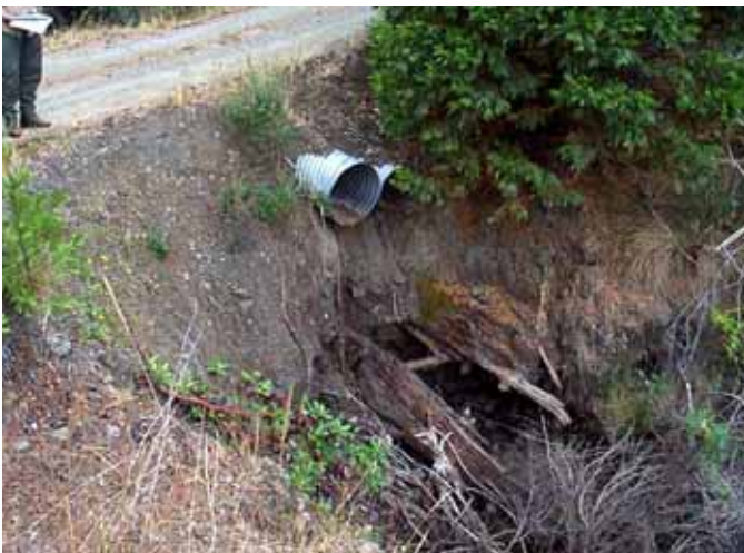
Figure 36. Watercourse crossing at high risk of failing.
