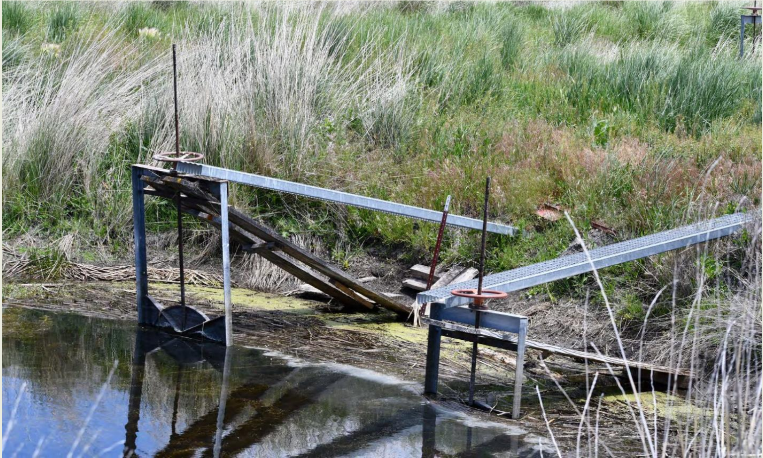
Failing set of screwgates, set at an incorrect elevation
