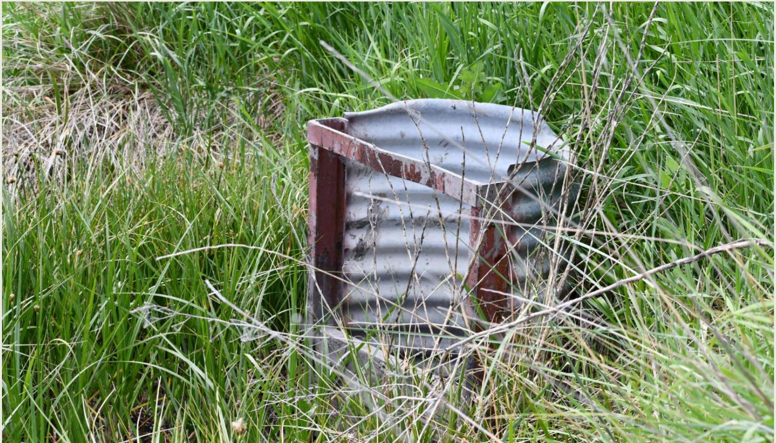
Dilapidated corrugated metal riser (water control structure)
