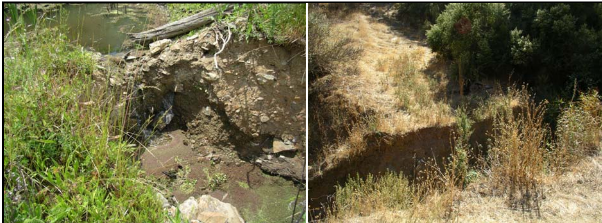
Figure 3. San Luis Reservoir Wildlife Area firebreak at Lost pond during early stages of erosion (at left, 2005) and after completely washed out with pond no longer dammed (at right, 2006).
