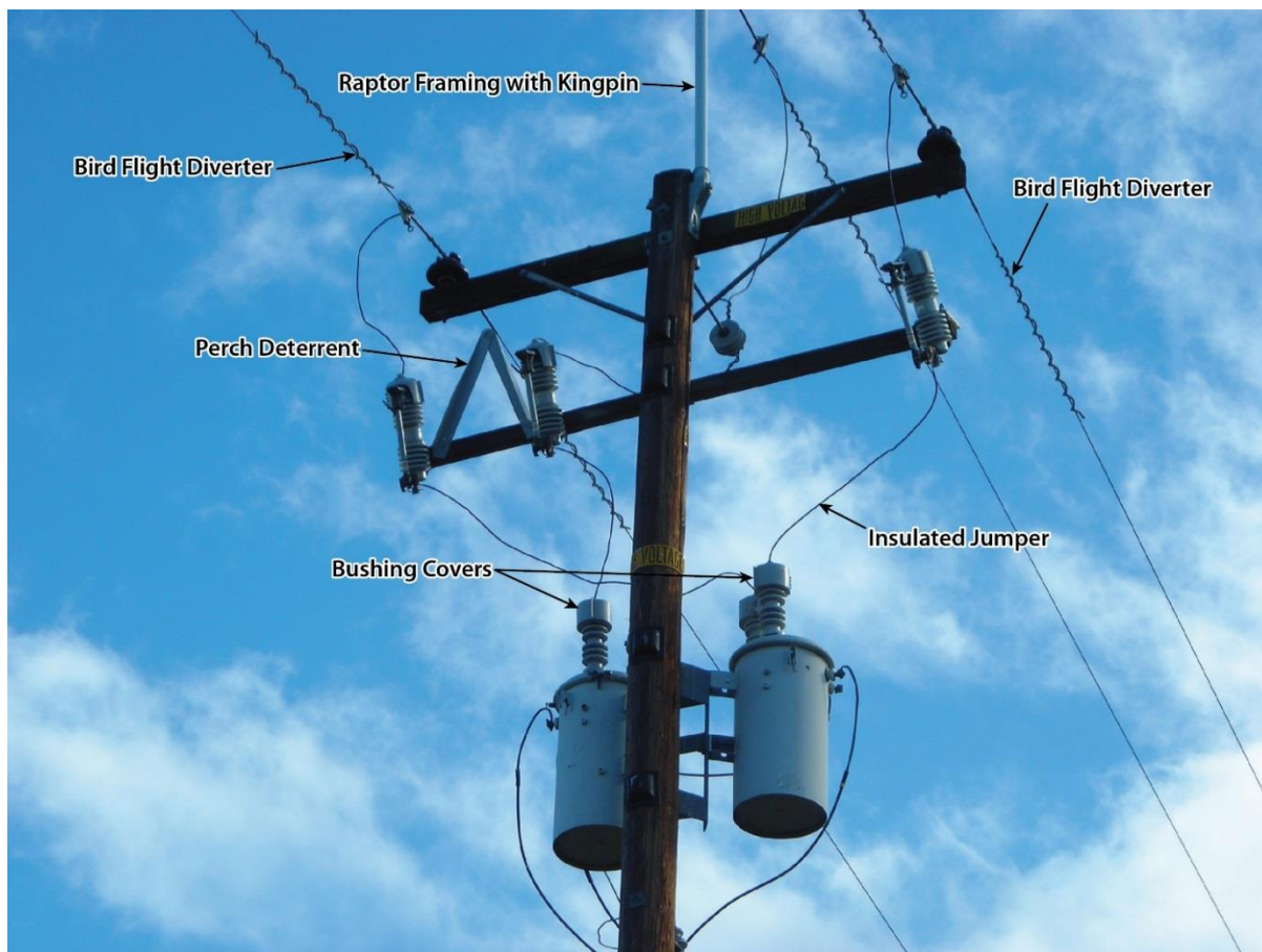
Figure 3. Important Avian Protection Hardware on Electric Facilities
