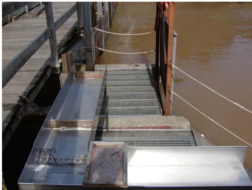
Figure 5. Pudding Creek fish ladder trap and flashboard dam. Stainless steel chute with water pump, fish holding tanks, grated walkways, lights, and safety lines are among the many improvements made to this structure as part of this study.
