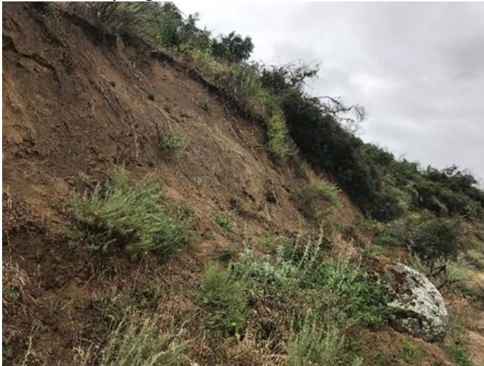
Slope failure at the entrance to the Reserve off Highway 78. Photo taken spring 2017, T. Stewart
