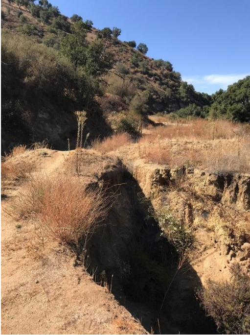
Above and below: Erosion and bike jump in Boden Canyon. Photos taken Oct. 2020. T Stewart
