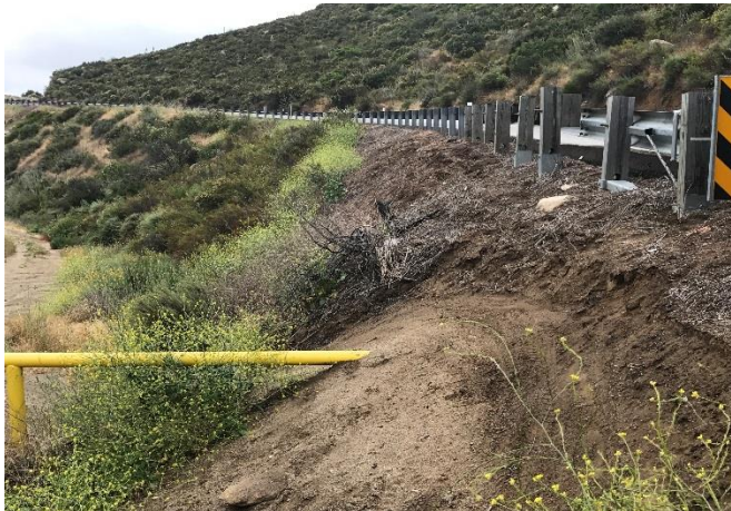
Erosion at gate caused by vehicular trespass, 2017. Photo by T. Stewart
