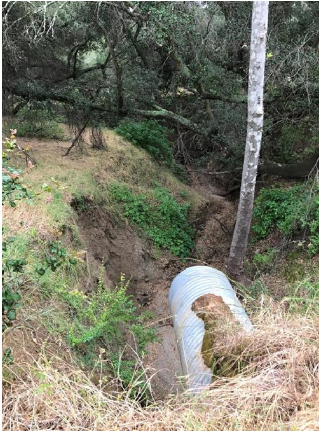
Culvert washout spring 2017, photo by T. Stewart
