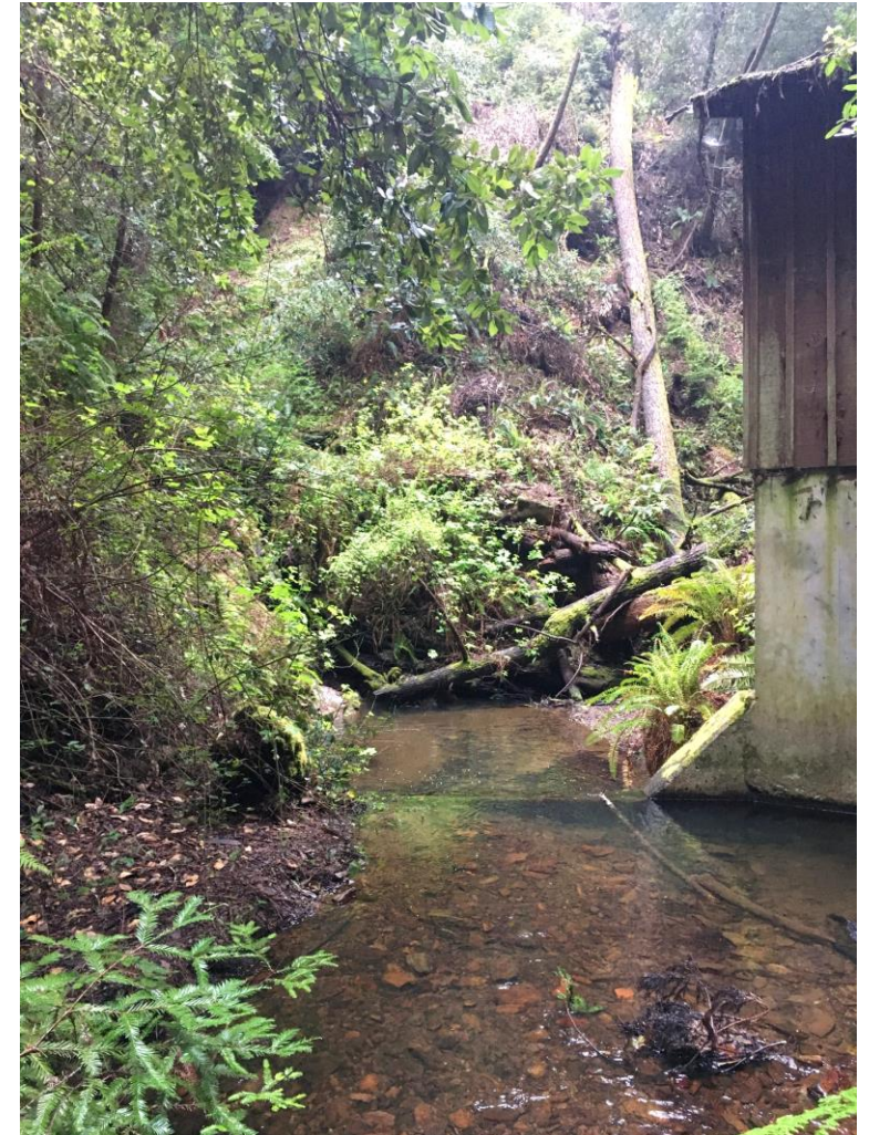
Point of diversion pre-fire looking downstream. The RCD and State Parks will replace this diversion as it was lost to the CZU fire.
