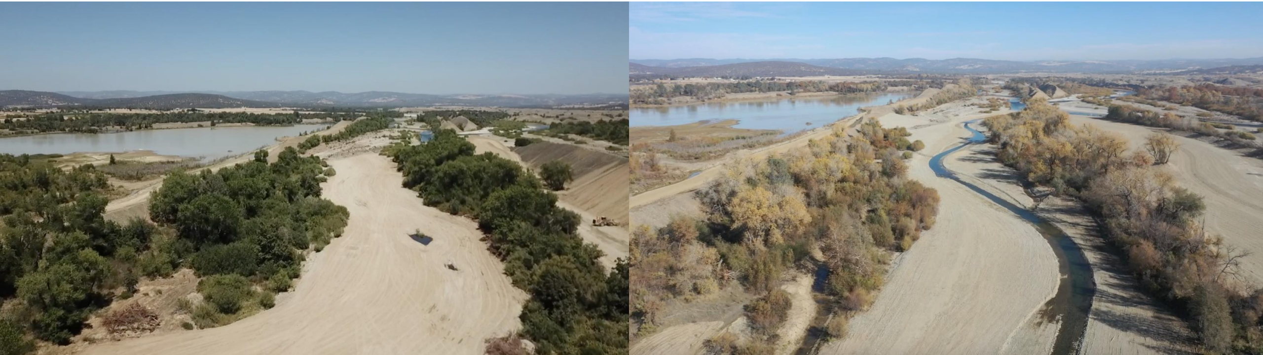
Phase I pre- (left) and post-fine (right) grading completed in 2020 at the perennial channel in the upper half of the site. Photo credit: CBEC Eco Engineering (Abe Aufdermauer)
