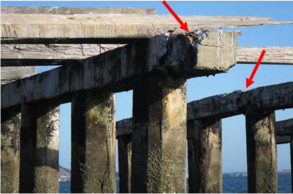
Photo 6: Typical Bent Cap Spalls
