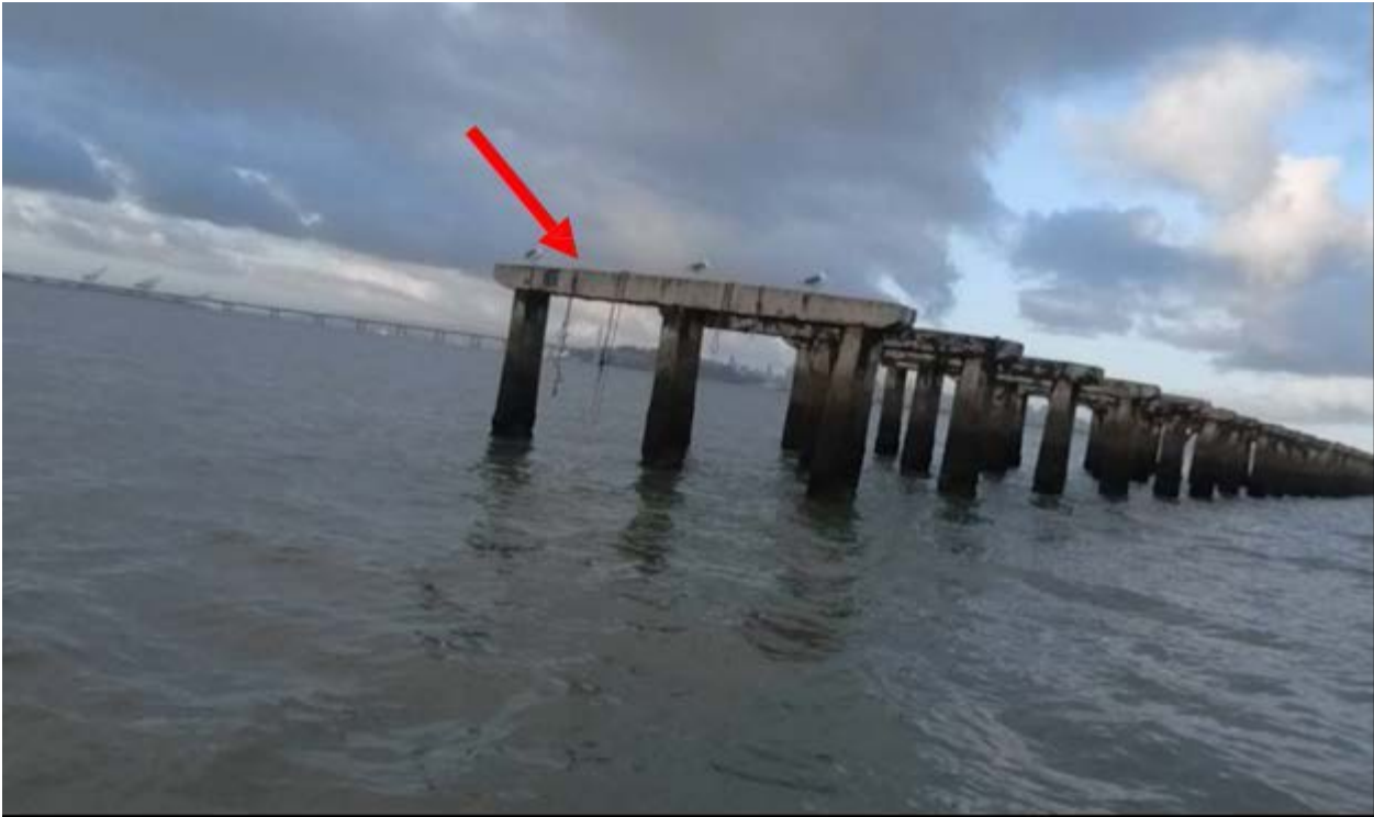
Photo 2: Multiple Rope Ladders Present at Section A
