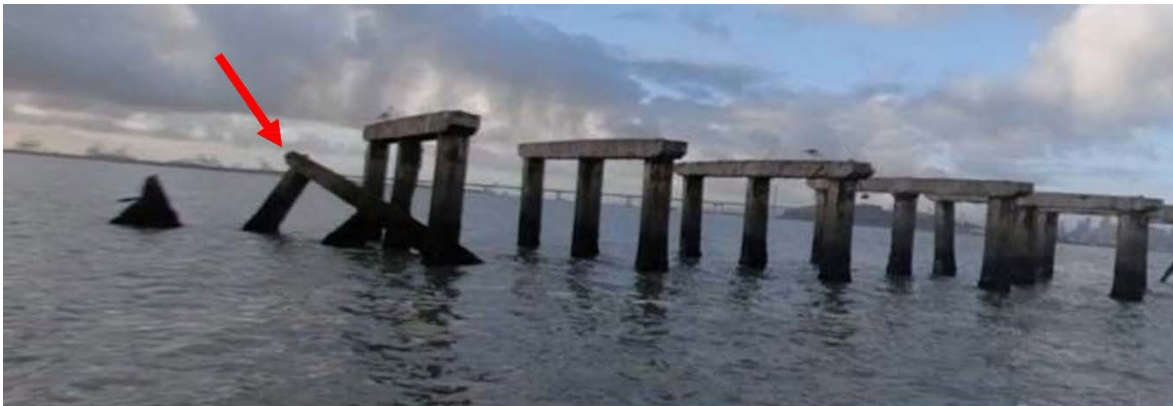
Photo 1: Example of Leaning Bent
