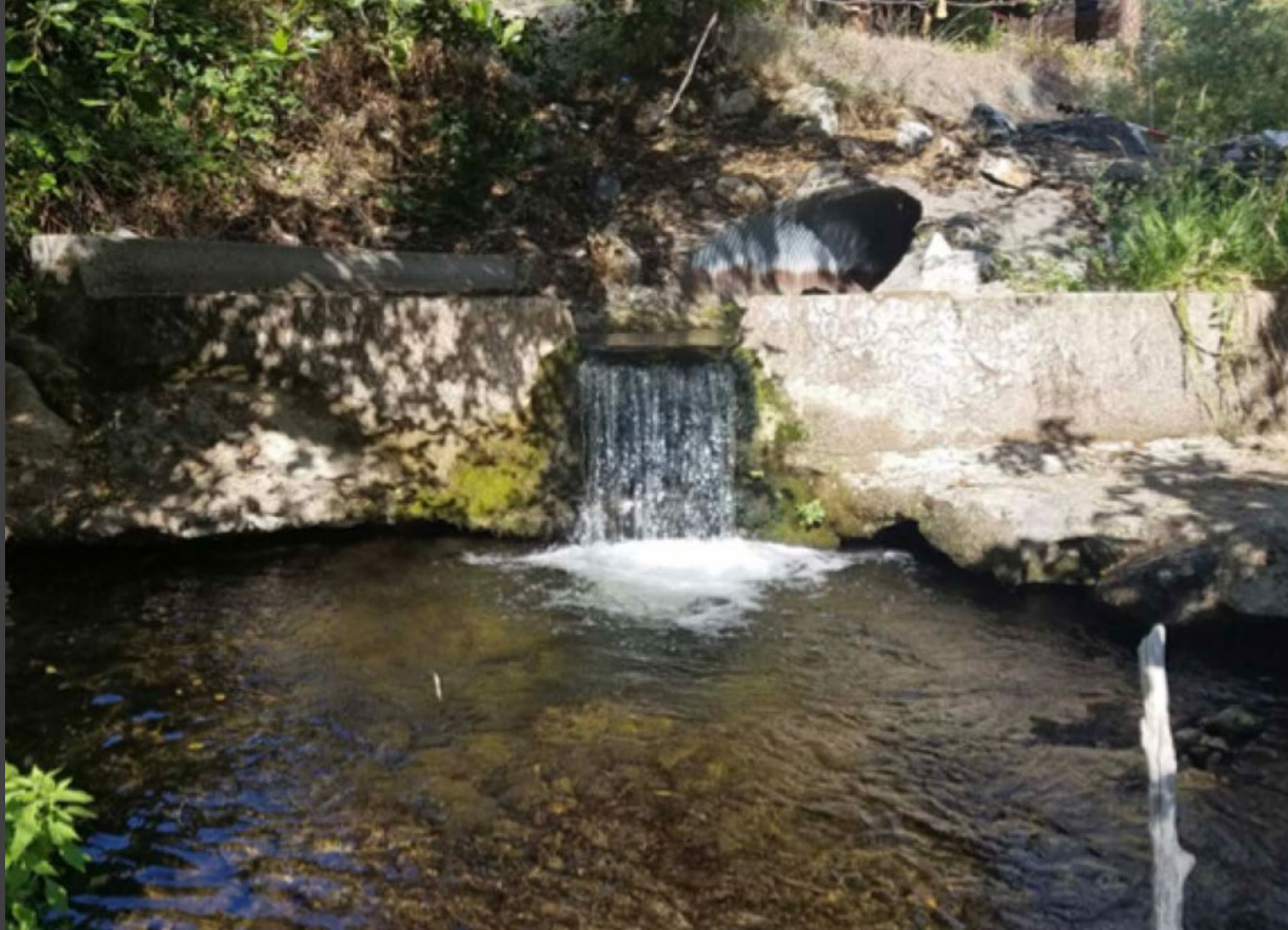
Fish Passage Barrier
