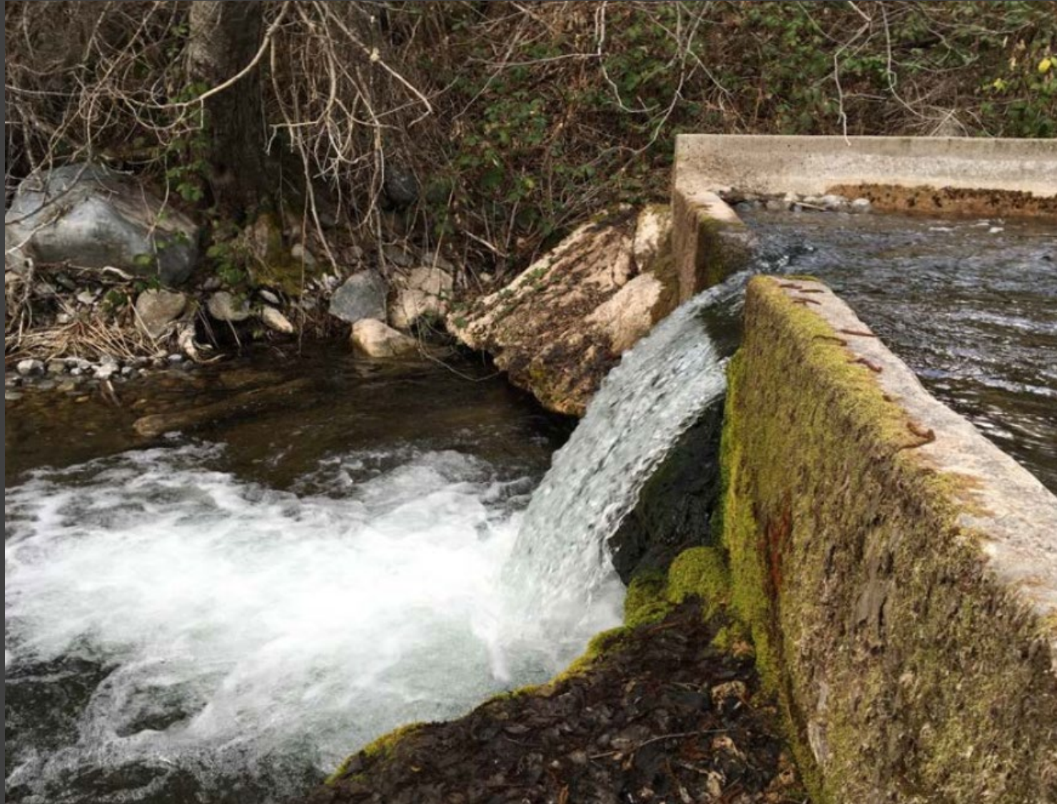
Fish Passage Barrier
