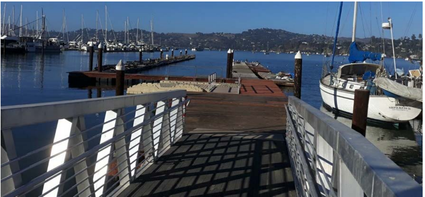
Image 1: This photo depicts the end of the main aluminum ramp and wooden docks that were supported by this grant. The black surface of the aluminum ramp is a fiberglass grate allowing sunlight to feed the eelgrass habitat under the ramp. The ramp connects to the lower wooden docks which have an inset with a plastic non-motorized small boat launch (ADA accessible by the smaller aluminum ramp). The small ramp and plastic ADA lower launch were funded by Water Trail Grant. Further away, the wooden dock extending to the right (south dock) was rebuilt with funds from this grant, as were portions of the left dock (north dock) and the perpendicular dock connecting the two main docks. Prior to the grant, we had no ramp to access the docks. Now we have a terrific and long lasting ramp that's ADA accessible (Photo credit: Sausalito Community Boating Center).
