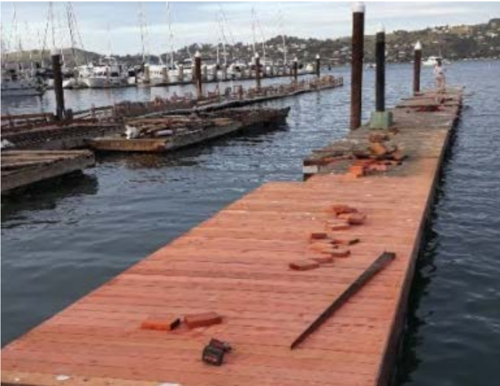
Image 10: Redwood decking installed on the south dock (Photo credit: Sausalito Community Boating Center).
