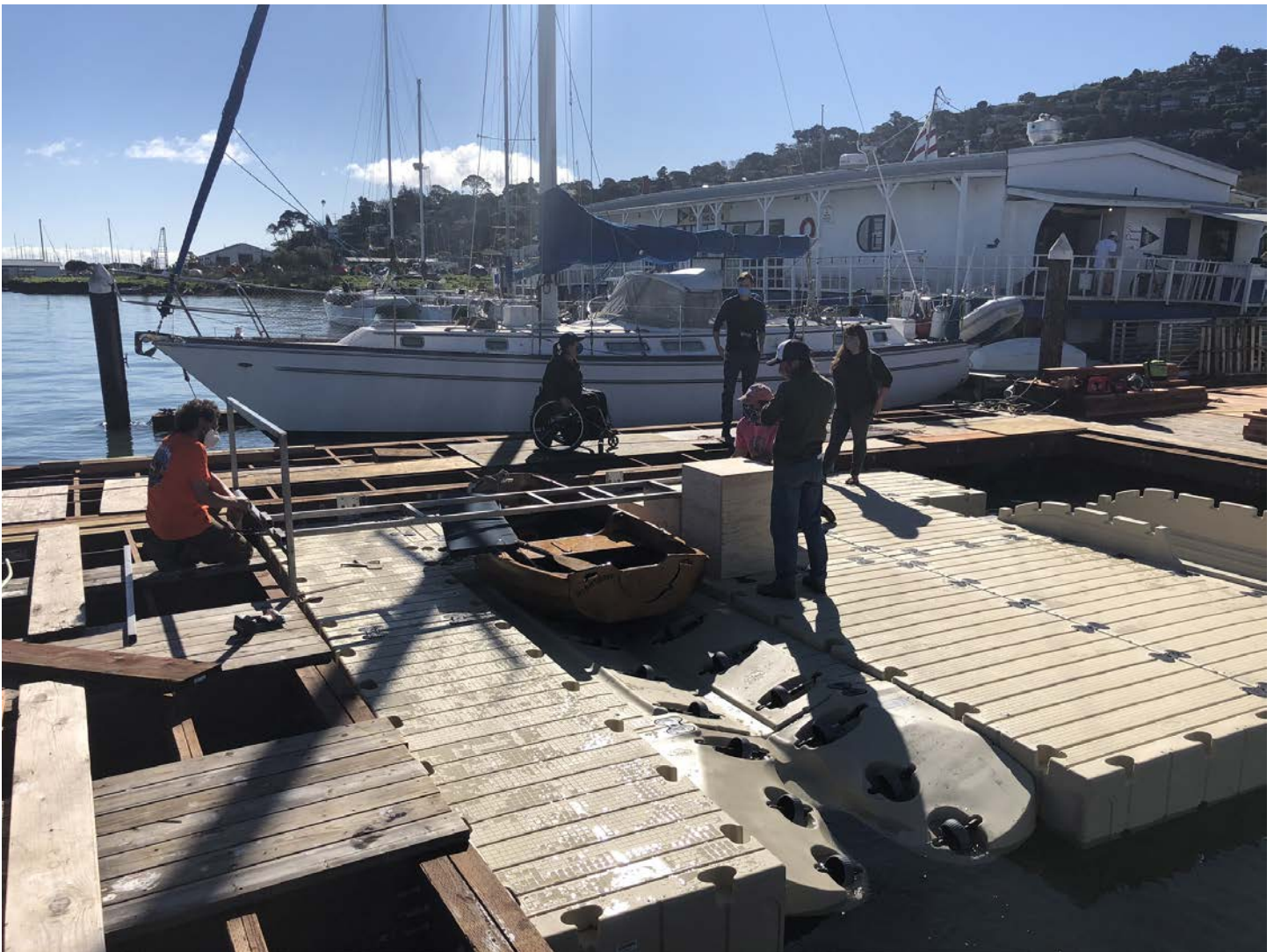
Image 3: This photo is a meeting of our ADA advisory group which brought in experts from the bay area disabled kayaking and sailing communities. They helped us design the lower plastic docks including the launching areas and a transfer bench system. This photo is while the project was a work in progress and the transfer bench (to transfer from wheelchair into kayak or small sailboat) was being completed. While funding from the NFWF and Cosco Busan Trustees were not applied directly to this aspect of the project, it was only because we received Cosco Busan funding that we were also able to complete this important aspect of our overall project design (Photo credit: Sausalito Community Boating Center).
