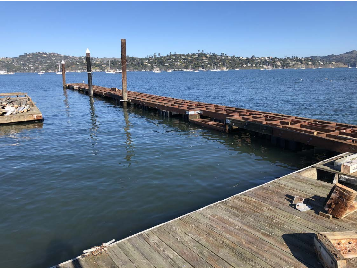
Image 9: South dock underlying infrastructure that was supported by this grant (Photo credit: Sausalito Community Boating Center).
