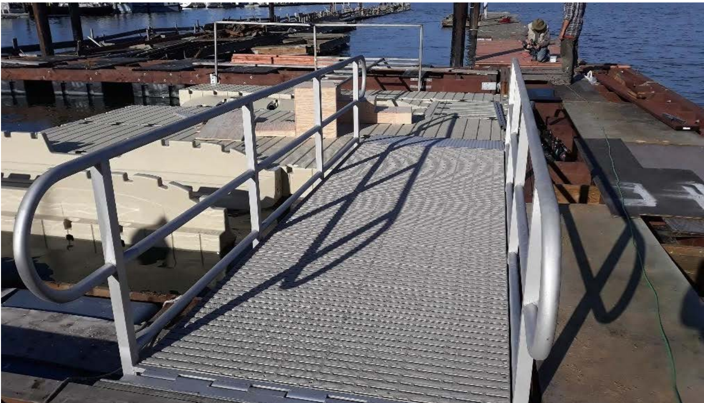
Image 6: Photo of smaller aluminum ramp installed to access lower plastic docks. Other wooden docks were under construction at the time of this picture (Photo credit: Sausalito Community Boating Center).
