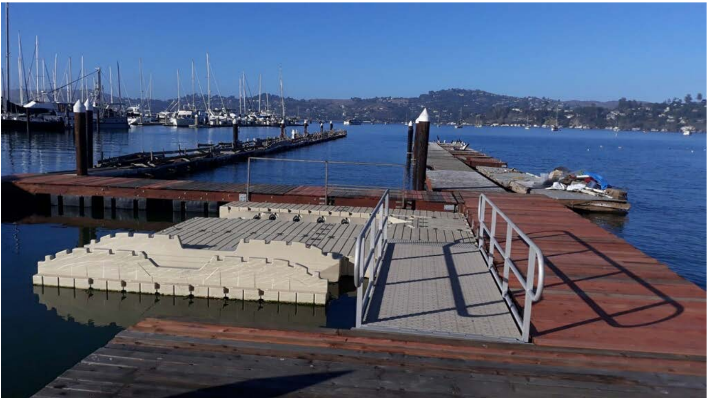
Image 7: The North docks on the right were nearly finalized at this point with electrical and plumbing installed underneath the decking. New redwood decking was installed along with the dock infrastructure being composed of redwood and supported by this grant. The south docks (to the left) have pinniped protections installed (Photo credit: Sausalito Community Boating Center).
