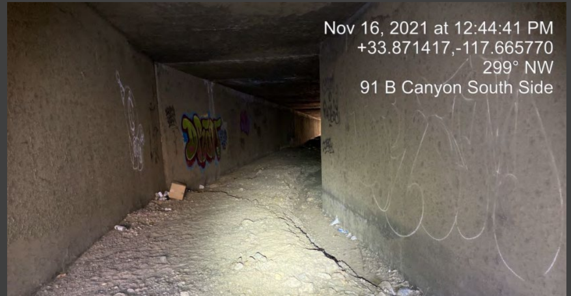
Kinked Culvert Under State Route 91
