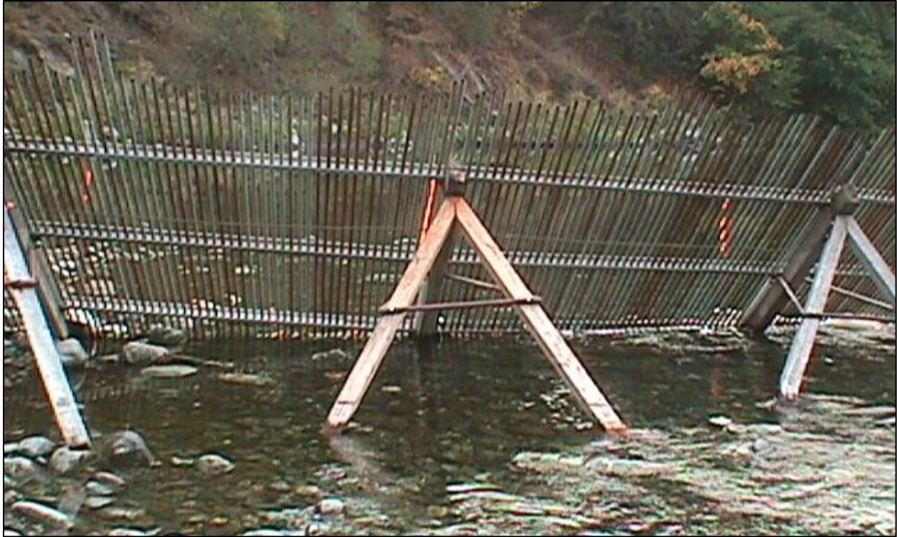
Figure 2. Photograph of Alaskan-style weir, tripods, support channels, and conduit (looking upstream).
