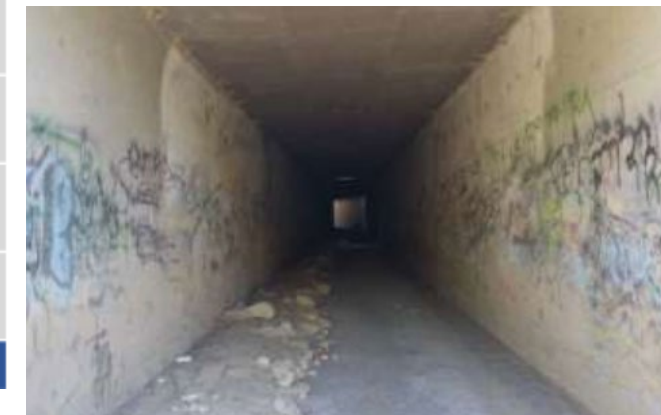
State Route 91 Kinked Culvert
