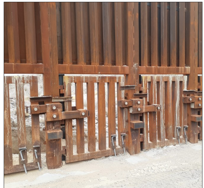
Photo 4. Flood gates built into the bollard fence at the bottom of most, but not all, drainages were to be unlocked and opened during flood events: however, all are welded shut.
