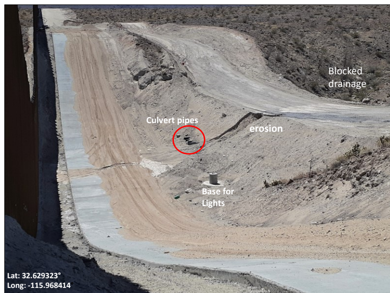
Photo 5. Construction road paralleling border fence destroyed vegetation and blocks all the drainages. Culvert pipes (red circle) are extremely small diameter and ineffective. Infrastructure for night-lighting is in place.
