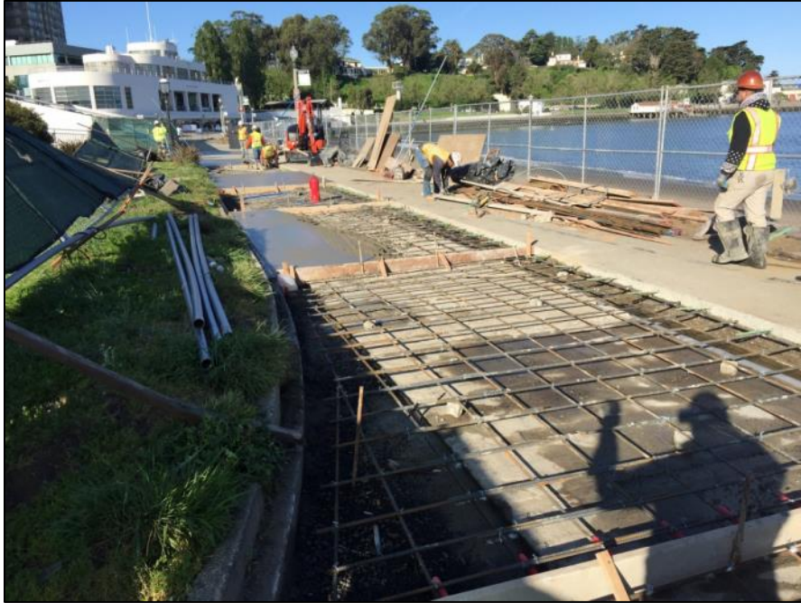
Figure 12. Aquatic Park Promenade rehabilitation – preparing the subgrade of subsided areas in order to resurface with concrete
