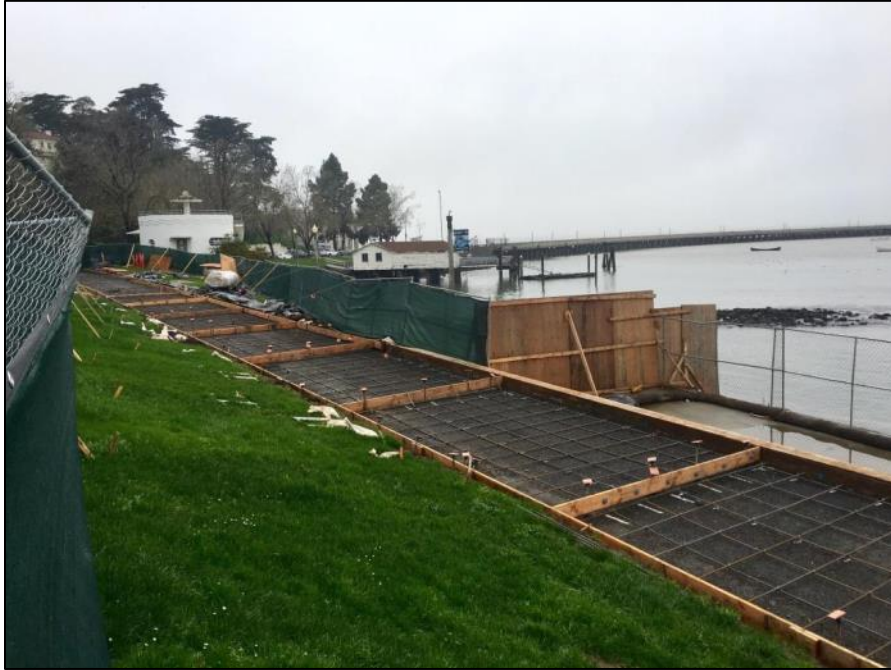
Figure 14. Rehabilitation of the Service Road that connects to Van Ness Avenue to meet accessibility standards – regraded and prepared for resurfacing the entire roadway with concrete
