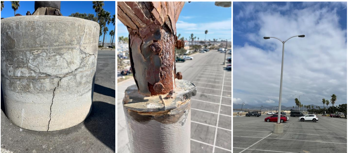
Project 2: "Before" photo of base of light pole at Harbor Cove Beach with cracks in it and need of replacement (left). "Before" photo of the top of one of the light poles at Harbor Cove Beach with significant rust and corrosion, and in need of replacement (center). "After" photo of one of the installed light posts at Harbor Cove Beach that are currently in use (right).
