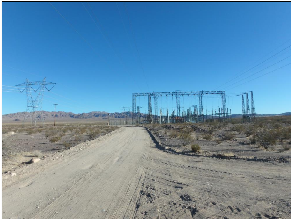
Figure 2. Current ground disturbances within the vicinity of the Project area, including an electrical substation. View north.
