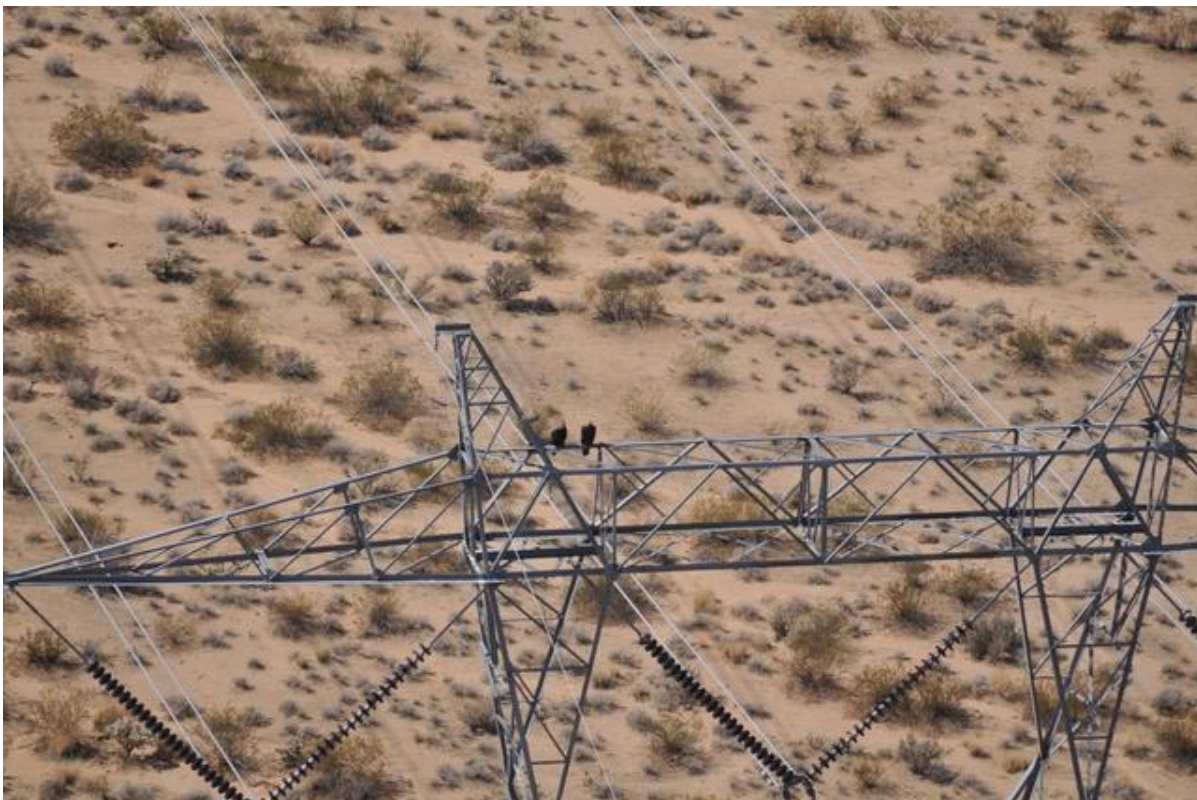
Photograph 4. Pair of golden eagles perched on a transmission structure.
